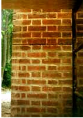
A mechanical grinder improperly used to cut out the horizontal joint and incompatible repointing have seriously damaged the 19th century brick. Photo: NPS files.
