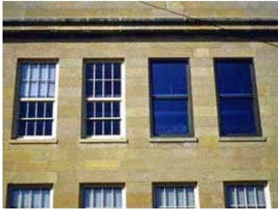
Tinted glazing has jeopardized the character of this historic office building and is, thus, not a recommended approach. Photo: Mike Jackson.
