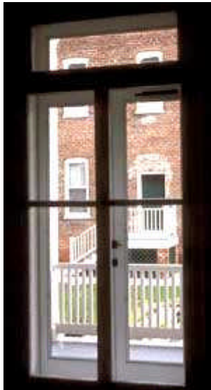
Storm doors have been added on the inside of this historic building as an energy-conserving device. Photo: NPS files.
