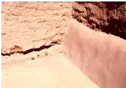
Coving at the base of this adobe wall may have been caused by salts deposited by rising groundwater and/or rainwater splash. Photo: NPS files.
