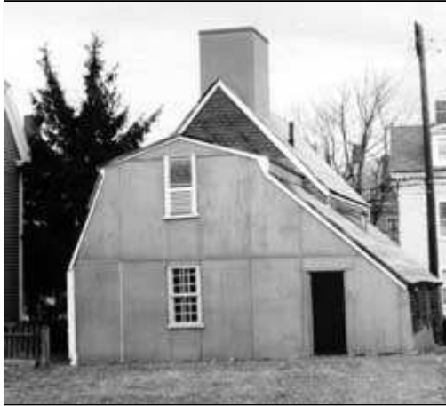
Temporary stabilization or "mothballing" with materials, such as plywood and building paper, can protect the roof of a project until it can be properly repaired or replaced. Photo: NPS files.
