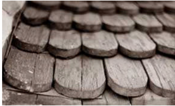
Replacement of particular historic details is important to the individual historic character of a roof, such as this rounded butt wood shingle roof. In the restoration, the drainage around a dormer was improved by the addition of carefully concealed modern metal flashing. Photo: NPS files.
