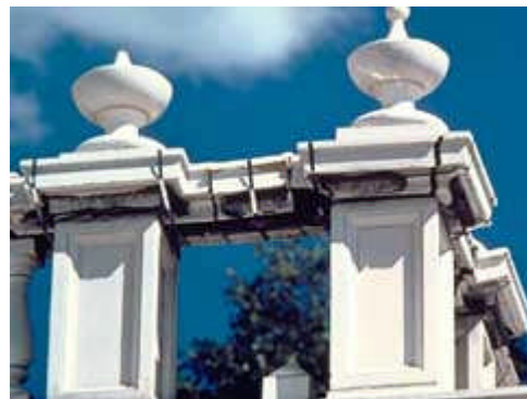
Exposed or freestanding terra-cotta detailing (parapets, urns, balusters, etc.) have traditionally been subjected to the most severe vicissitudes of deterioration as a result of freezing temperatures and water. Photo: NPS files.
