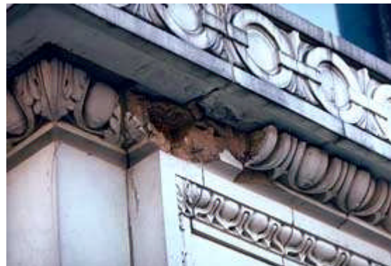
Material spalling is the result of excessive expansion of the porous tile body caused by water and freezing temperatures. This is a serious condition, often difficult to repair. Photo: NPS files.
