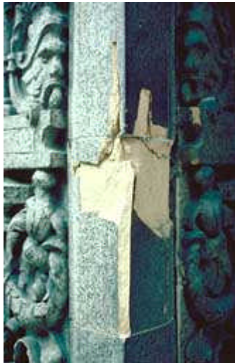
The damage shown here is the result of direct live load on a mid-rise building. The steel frame has settled and shifted the weight onto the exterior terra-cotta cladding, resulting in rupturing of the material. Photo: NPS files.
