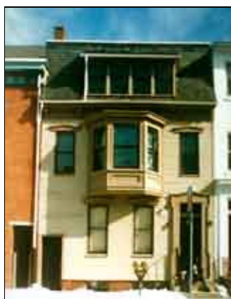
In this successful residential rehabilitation, deteriorated wood siding was removed from the foundation to the top of the first floor windows and replaced with matching wood siding. The
