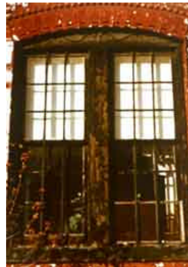
Deteriorating operable windows often contribute to lead dust in a house. In homes with small children, floors and other surfaces should be kept as clean as possible to avoid lead contamination.
