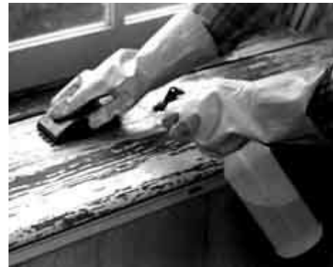
Wet sanding of interior surfaces will keep lead dust levels down, reduce the need for workers' protection, and provide a sound surface for repainting. Photo: NPS files.
