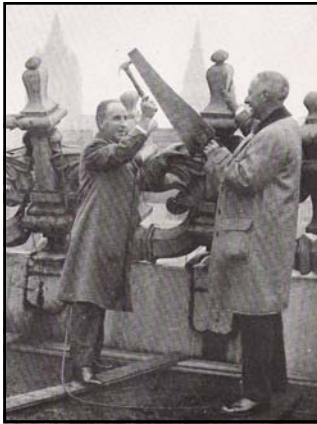
JJ Raskob & Al Smith ceremoniously begin the mighty task of demolishing the Waldorf-Astoria Hotel
