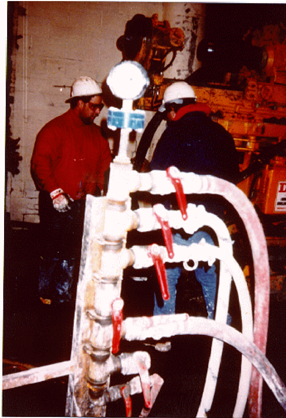
Figure 8-6. Drill Rig Pressure Gauge.
