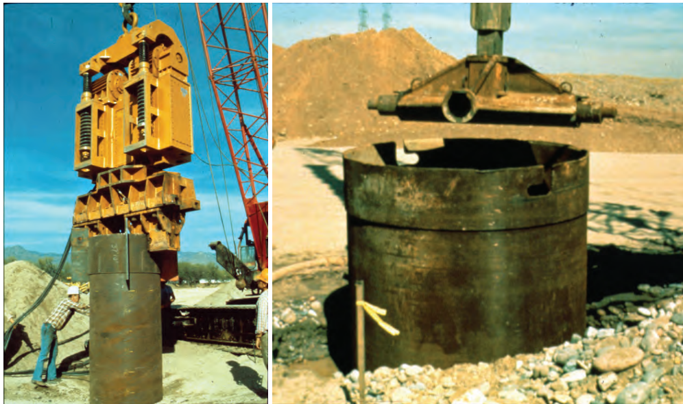
Figure 4-10 Use of a Vibro-Hammer (Left) and Twister Bar (Right) to Advance Casing
