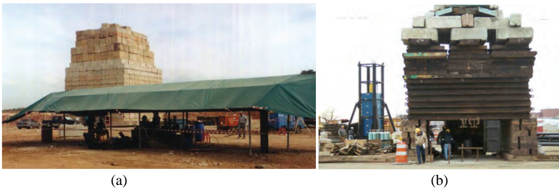
Figure 17-1 Kentledge Static Load Tests with (a) Bi-directional (O-cell) Test; (b) Rapid Load Test (Statnamic) (photos courtesy Loadtest, Inc. and Applied Foundation Testing)
