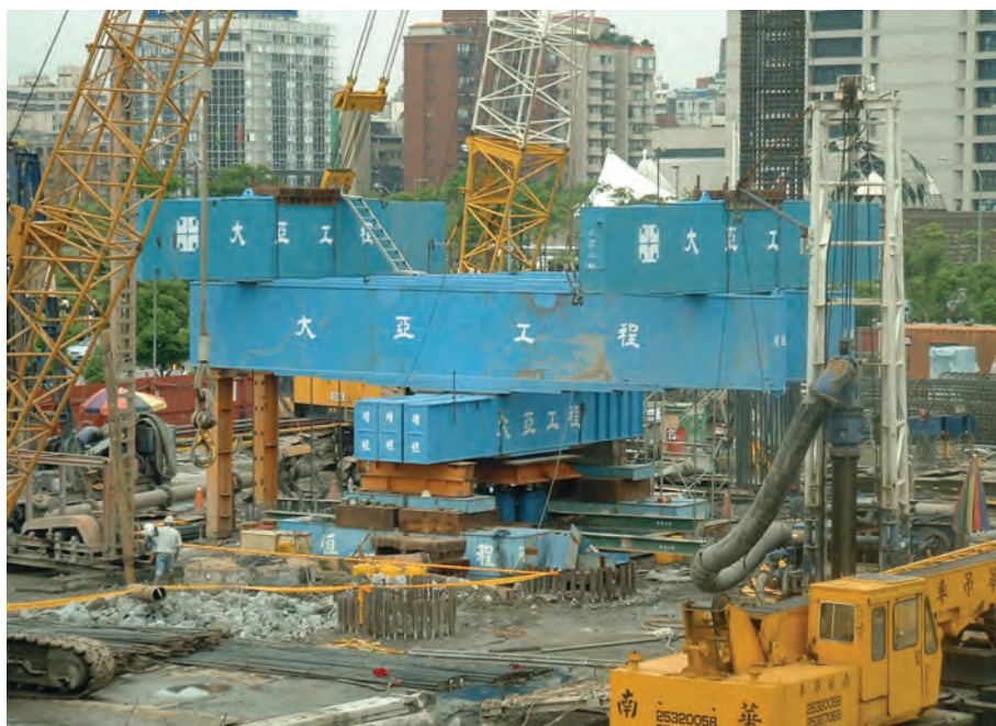
Figure 17-11 5,700 ton Capacity Load Test in Taiwan (photo courtesy Prof. San-Shyan “Sonny” Lin)
