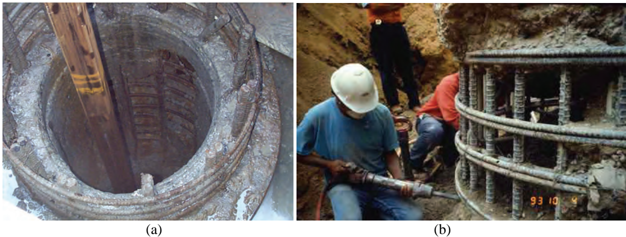
Figure 21-7 Excavation and Replacement of Defective Concrete Using (a) Drilling Tool within the Cage and (b) Hand Methods (photos courtesy Caltrans)
