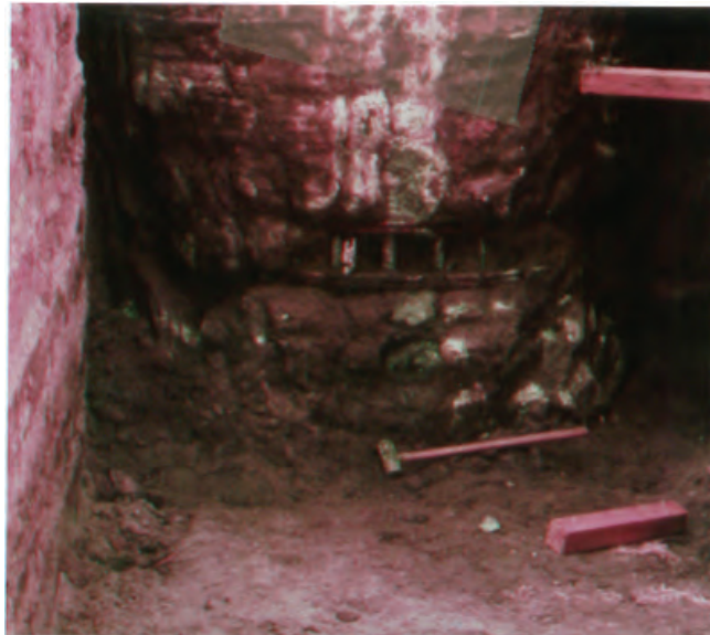
Figure 20-9 Defect Similar to the Defect that Produced the Logs in Figure 20-8 (Courtesy of Caltrans)
