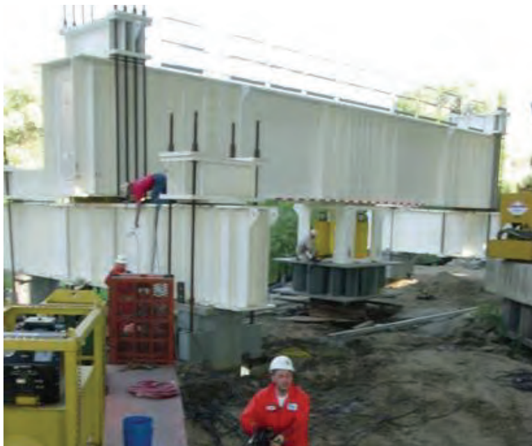
Figure 17-10 4,000 ton Capacity Reaction System (photo courtesy of Caltrans)
