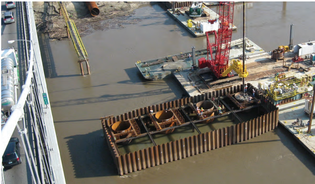
Figure 1-9 Construction of 12-ft Diameter Drilled Shafts for the Main Pylon Foundation, Christopher S. Bond Bridge, Kansas City (photo by Gary Naugle, MoDOT)
