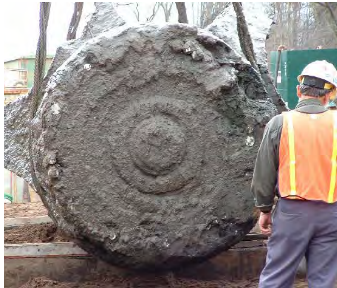
Figure 9-16 Exposed Bottom Surface of an Exhumed Drilled Shaft
