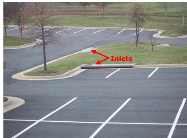
Two Curb-Opening Inlets at Low Spots
