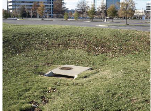
A Dry Pond with Storm Sewer
