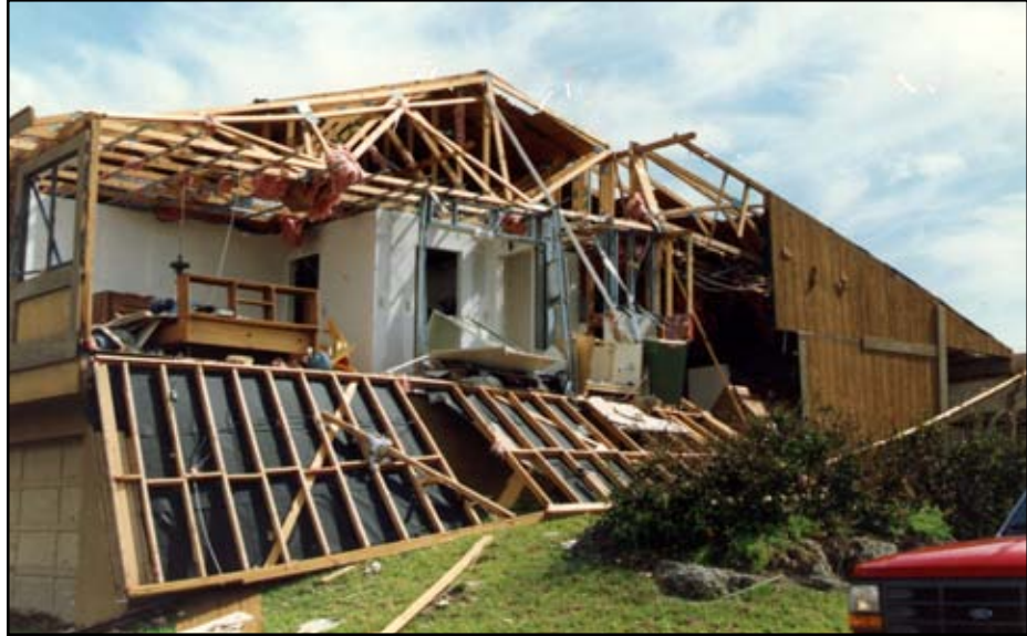
Figure 7-24 Hurricane Andrew (1992). End-wall failure of typical first-floor masonry/second- floor wood-frame building in Dade County, Florida.
