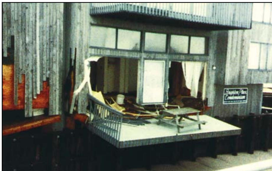
Figure 7-15 Damage to oceanfront condominium in Ocean City, New Jersey, caused by wave runup on a timber bulkhead. April 1984 photograph by Mark Mauriello.
