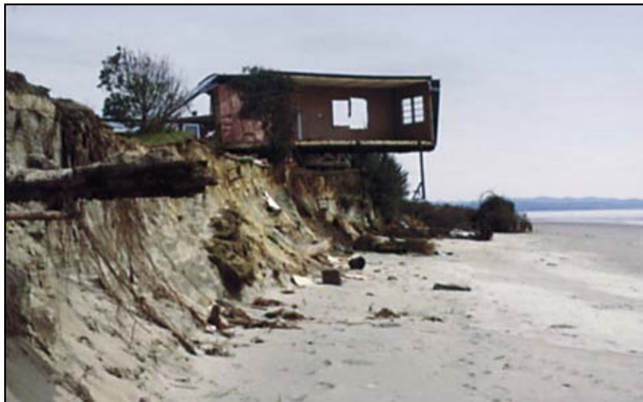
Figure 7-30 Erosion undermining a coastal residence at Cape Shoalwater, Washington. 1992 photograph by Washington Department of Ecology.
