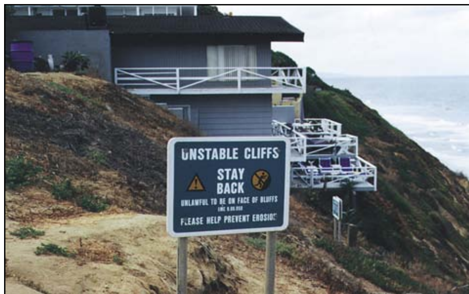
Figure 7-56 Unstable coastal bluff at Beacon's Beach, San Diego, California. Photograph by Lesley Ewing.
