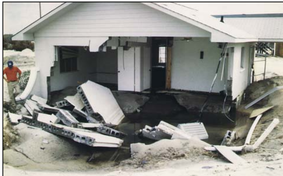
Figure 7-52 Hurricane Fran (1996). Extreme case of localized scour undermining a slab-on-grade house on Topsail Island, North Carolina. The lot was several hundred feet from the shoreline and mapped as an A zone on the FIRM prior to the storm. This case provides one argument for the treatment of these areas as coastal A zones.
