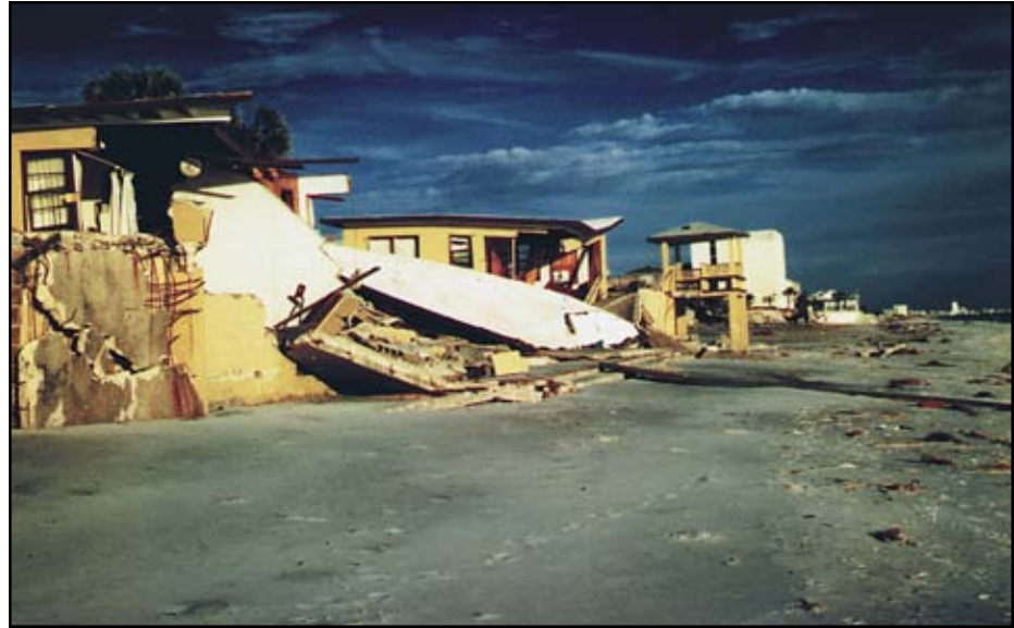
Figure 7-28 Hurricane Opal (1995). Failure of seawall in Bay County, Florida, led to undermining and collapse of the building behind the wall.
