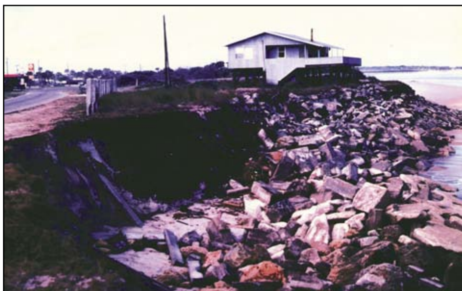
Figure 7-27 Erosion and revetment damage in St. Johns County, Florida, caused by the November 1984 northeast storm.
