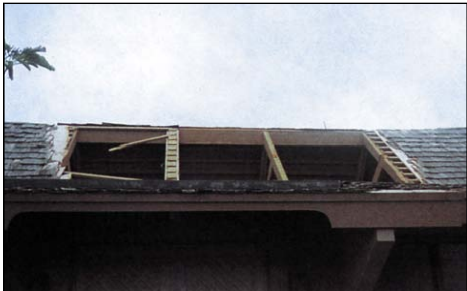
Figure 7-25 Hurricane Iniki (1992), Kauai County, Hawaii. Loss of roof sheathing due to improper nailing design and schedule.
