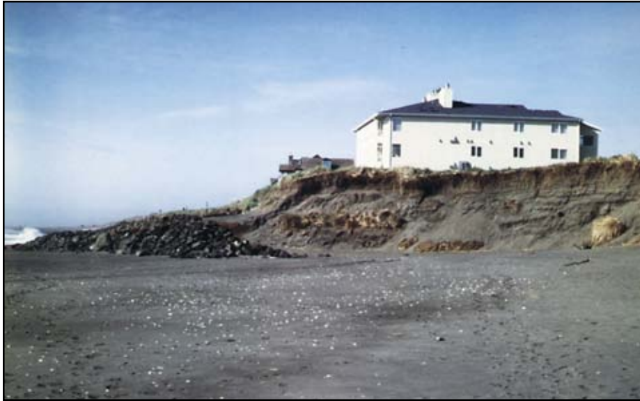
Figure 7-46 Buildings threatened by erosion at Ocean Shores, Washington. The rock revetments were built in response to shoreline erosion along an area adjacent to a jetty and thought to be accretional. 1998 photograph.
