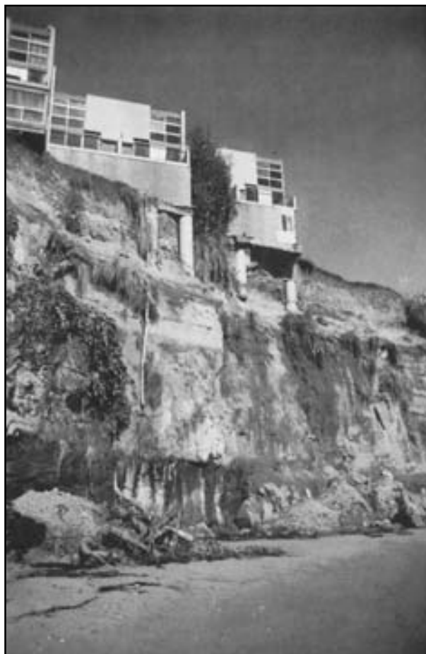
Figure 7-39 Bluff failure by a combination of marine, terrestrial, and seismic processes led to progressive undercutting of blufftop apartments at Capitola, California. Six of the units were demolished after the 1989 Loma Prieta earthquake. 1989 photograph from Griggs (1994), courtesy of Journal of Coastal Resources.
