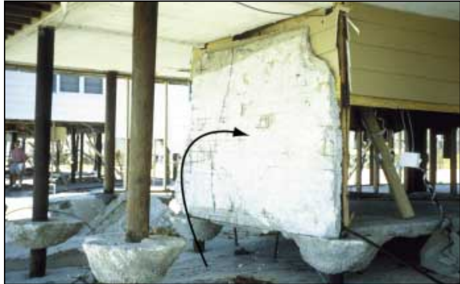
Figure 7-16 Hurricane Fran (1996). Concrete slab-on-grade flipped up by wave action came to rest against two foundation members, generating large unanticipated loads on the foundation.
