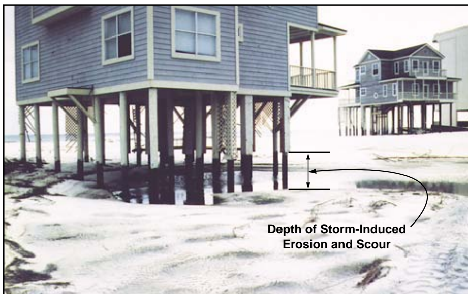
Figure 7-11 Pile-supported house in the area of channeled flow shown in Figure 7-10. The building foundation and elevation successfully prevented high-velocity flow, erosion, and scour from destroying this building.
