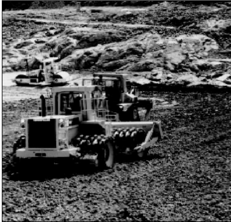
Figure 18, Earth fill (zone 1) compaction by a model 925 C Caterpillar pad foot roller.
