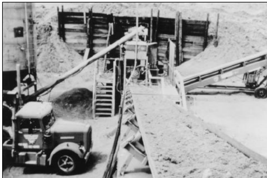
Figure 46, Cement vane feeder and soil feed belt to pugmill.
