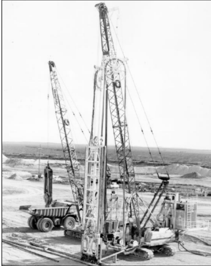
Figure 11, Slurry wall construction using panel excavation and tremie placement, view of a hydromill and crane with 30-inch x 10-ft clamshell.
