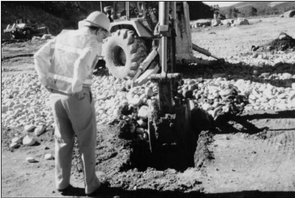
Figure 27, Test pit at the interface of a sand filter and gravel drain.
