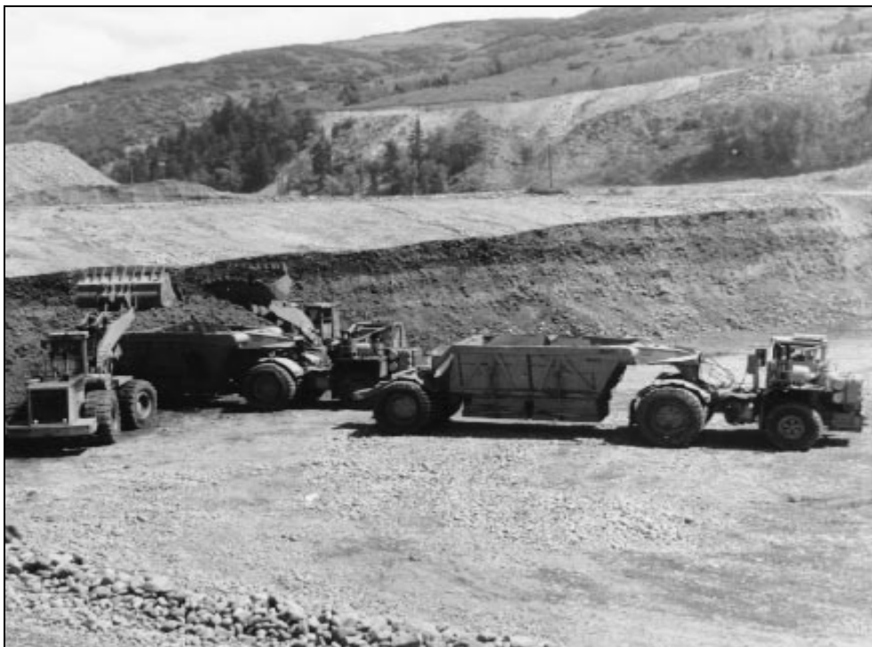
Figure 25, Two model 992C Caterpillar front end loaders loading zone 4 (gravel and cobble fill) from borrow into a model 540 Dart belly dump truck.
