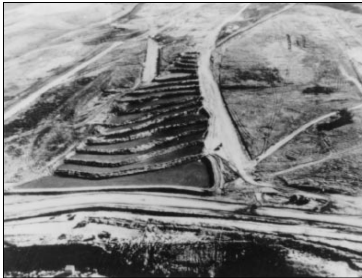
Figure 9, Ponding dry foundation of a Dam in Nebraska.
