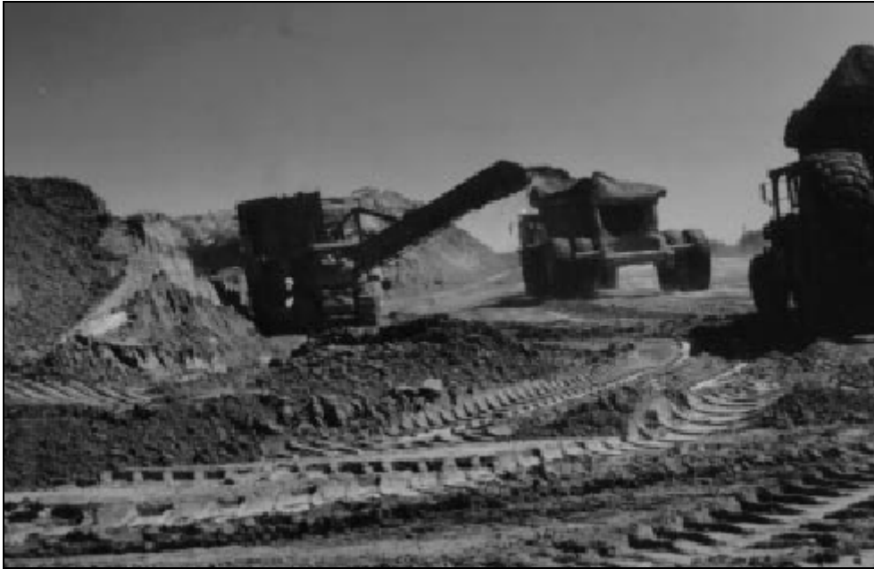
Figure 24, A Holland loader excavating a vertical face mixing silt and fine sand deposits for impervious fill.
