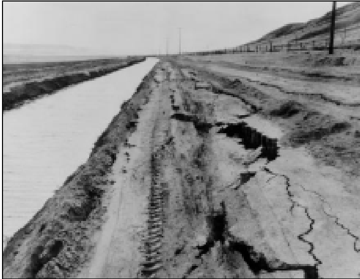
Figure 8, Cracking and settling of canal bank in dry, low-density silt.
