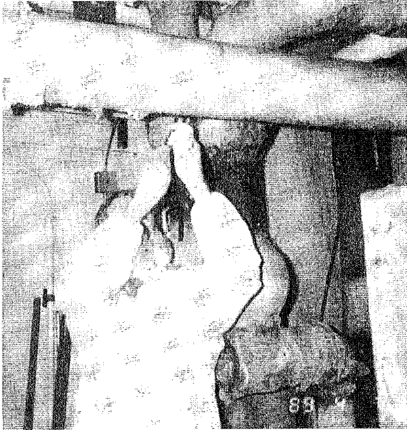
A properly trained and protected building inspector collecting a bulk sample of suspected asbestos-containing thermal system insulation.
