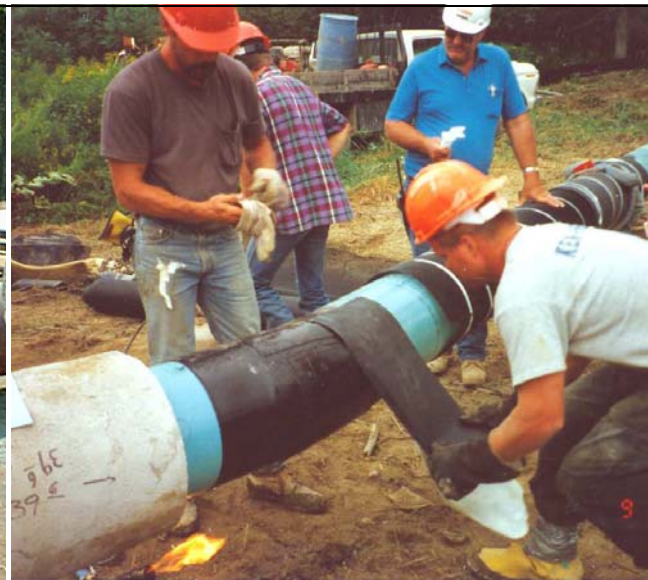
Figure 26: Application of Heat-Shrink Sleeve - Wrapping of Pipe with Sleeve in an Overlapping Pattern
