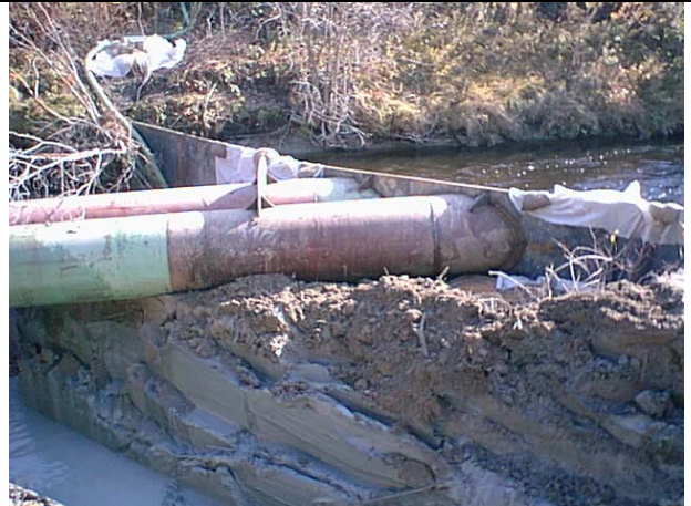
Figure 37: Functioning Dual Flume Assembly - River Entering Flumes (upper right) - Excavated Pipeline Trench (lower left)
