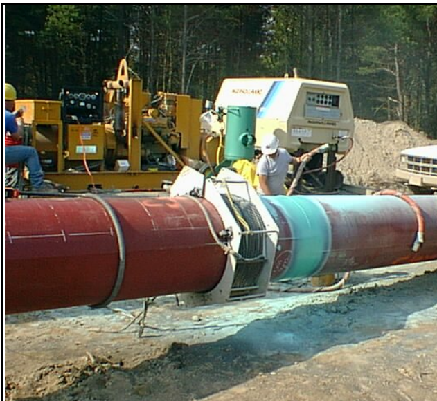
Figure 25: Application of Fusion Bond Epoxy - Cooling Heat Ring (left of center) and Finished Field Coating (right of center)
