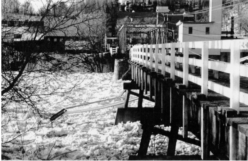
Figure 1-4. Ice action on bridge piers
