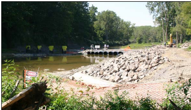
Figure 3-46. Cazenovia Creek ICS under construction September 2005, showing the rock berm along the right bank.
