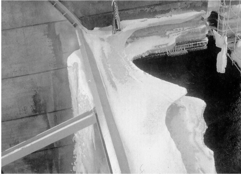
Figure 1-2. Ice accumulation on dam gates
