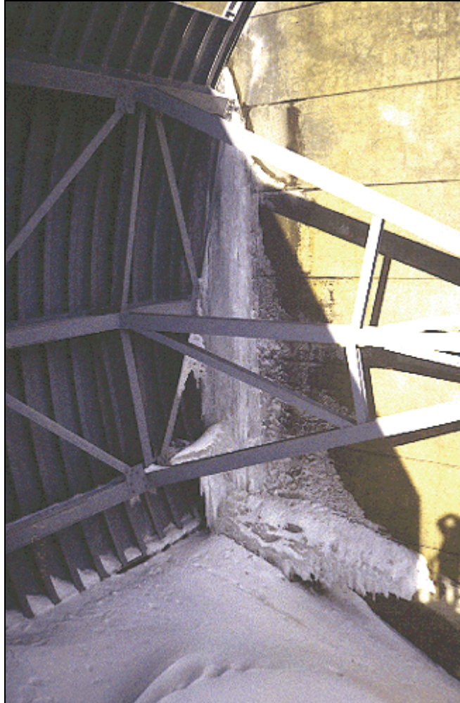
Figure 20-1. Column of ice formed on the downstream side of a tainter gate from water leaking past the side seal. The ice forms a bridge between the gate and pier. Such accumulations prevent movement of the gate. To restore normal gate operations, the ice needs to be removed by melting, chipping, or cutting. Photo of Gavens Point Dam, Yankton, SD.
