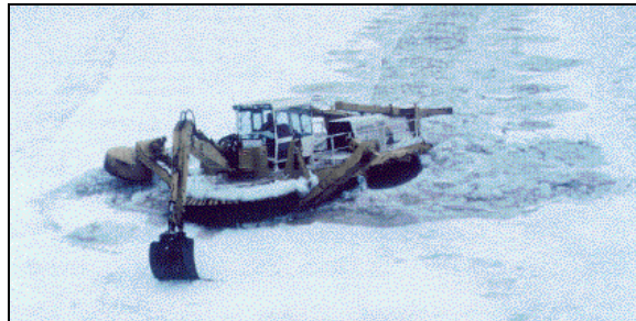
Figure 3-11. Breaking ice with an amphibious excavator on the Aroostook River, Ft. Fairfield, Maine.
