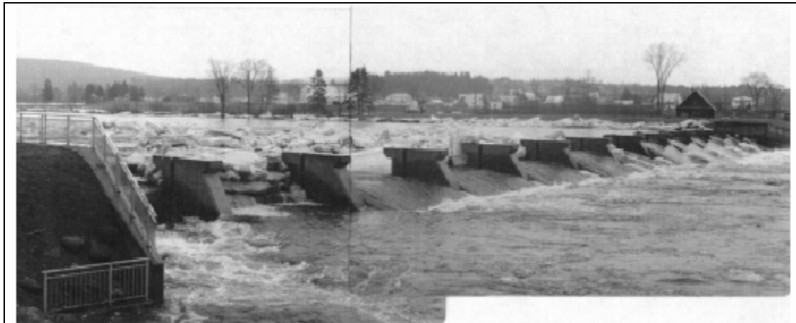
Figure 3-37. Weir with piers ice control structure on the Ste. Anne River, St. Raymond, Quebec. (Photo courtesy of Marc Delagrave, Roch Itée Groupe-conseil, Sainte-Foy, Quebec.)
