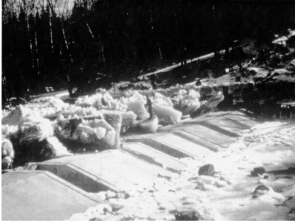
b. Ice accumulated behind structure in early spring
