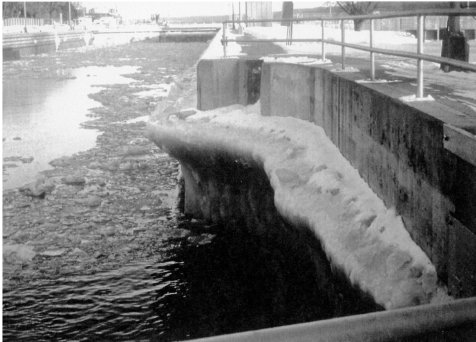
Figure 1-3. Ice collar on lock wall
