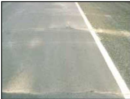
FIGURE 46 Distress Type ACP 15—Fine Material Left on Surface by Water Bleeding and Pumping
