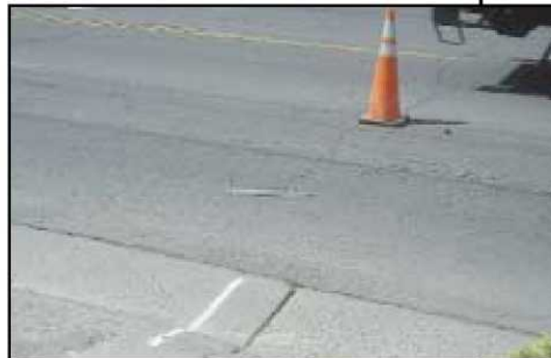
FIGURE 20 Distress Type ACP 6—Moderate Severity Transverse Cracking
