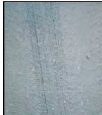
FIGURE 38 Distress Type ACP 11— Aggregate Obscured
