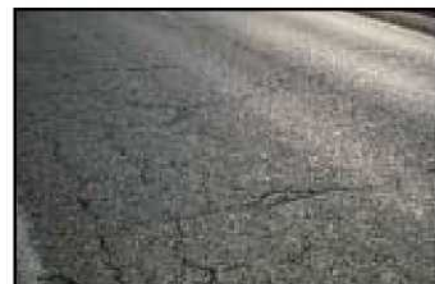
FIGURE 10 Distress Type ACP 2—High Severity Block Cracking
