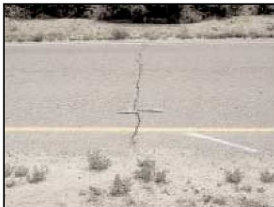
FIGURE 21 Distress Type ACP 6—High Severity Transverse Cracking
