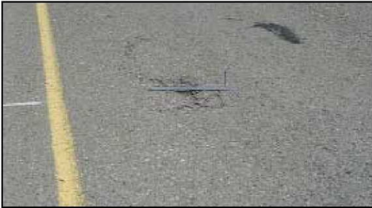
FIGURE 27 Distress Type ACP 8—Low Severity Pothole
