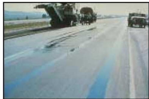
FIGURE 33 Distress Type ACP 9—Standing Water in Ruts
