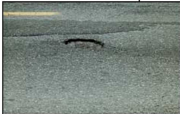
FIGURE 28 Distress Type ACP 8—Moderate Severity Pothole
