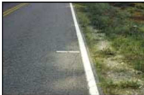
FIGURE 12 Distress Type ACP 3—Low Severity Edge Cracking
