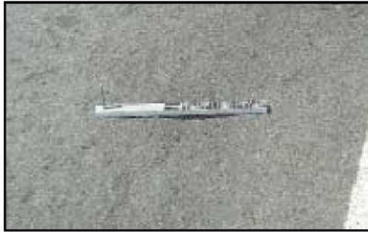
FIGURE 40 Distress Type ACP 13—Loss of Fine Aggregate
