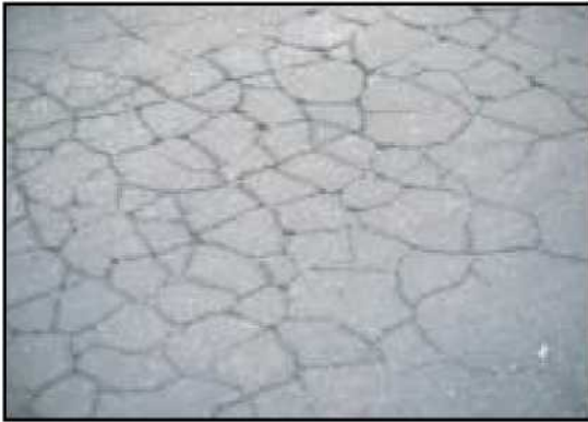
FIGURE 4 Distress Type ACP 1—Chicken Wire/Alligator Pattern Cracking Typical in Fatigue Cracking
