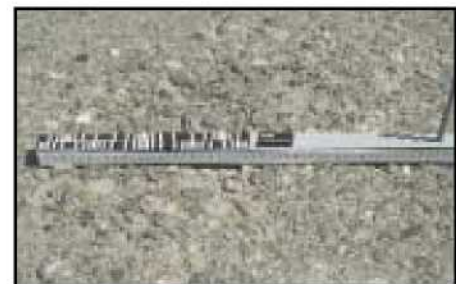
FIGURE 42 Distress Type ACP 13—Loss of Coarse Aggregate
