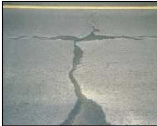
FIGURE 45 Distress Type ACP 15—Water Bleeding and Pumping
