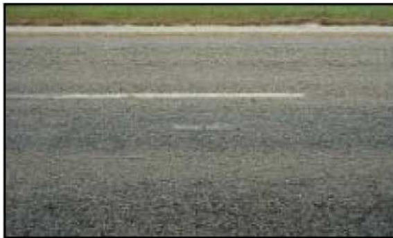
FIGURE 36 Distress Type ACP 11—Discoloration
