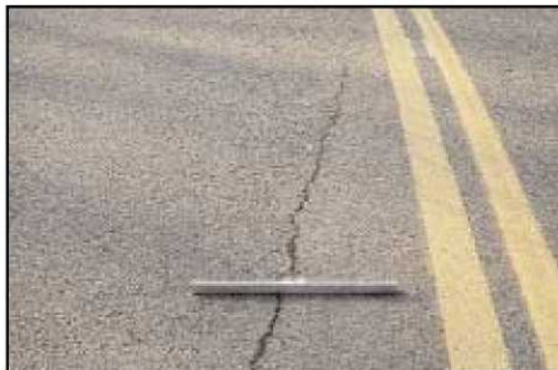
FIGURE 15 Distress Type ACP 4b—High Severity Longitudinal Cracking not in the Wheel Path
