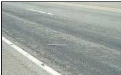
FIGURE 37 Distress Type ACP 11—Loss of Texture
