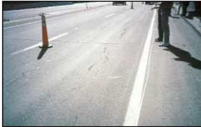
FIGURE 5 Distress Type ACP 1—Low Severity Fatigue Cracking
