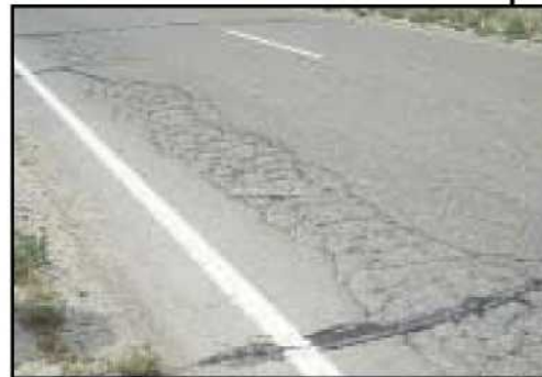
FIGURE 7 Distress Type ACP 1—High Severity Fatigue Cracking with Spalled Interconnected Cracks
