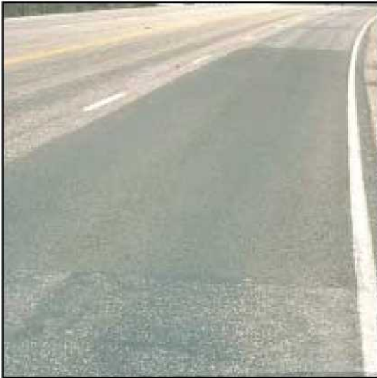
FIGURE 23 Distress Type ACP 7—Low Severity Patch
