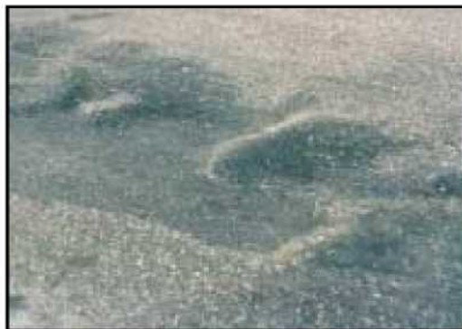
FIGURE 35 Distress Type ACP 10—Shoving in Pavement Surface
