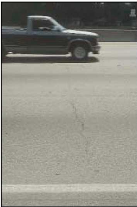
FIGURE 19 Distress Type ACP 6—Low Severity Transverse Cracking
