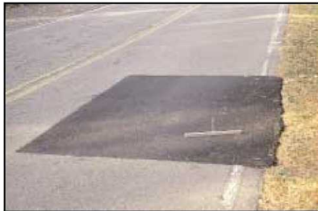
FIGURE 24 Distress Type ACP 7—Moderate Severity Patch
