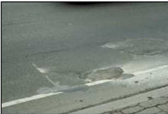
FIGURE 25 Distress Type ACP 7—High Severity Patch
