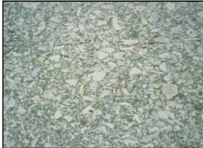
FIGURE 39 Distress Type ACP 12—Polished Aggregate
