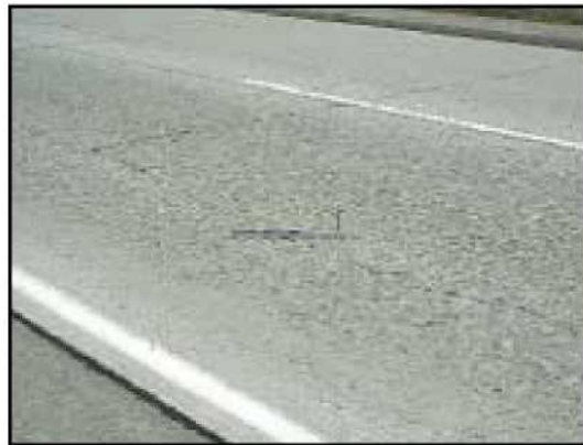
FIGURE 56 Distress Type JCP 3—Moderate Severity Longitudinal Cracking
