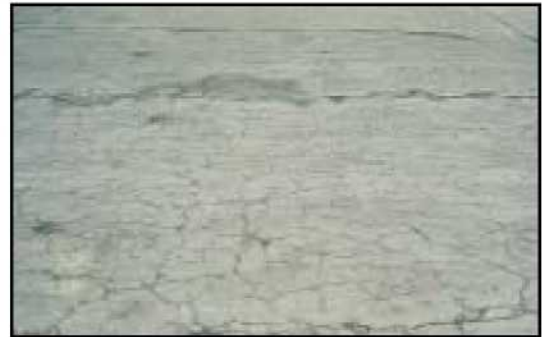
FIGURE 69 Distress Type JCP 8a—Map Cracking
