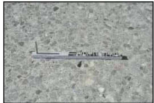
FIGURE 74 Distress Type JCP 10—A Popout
