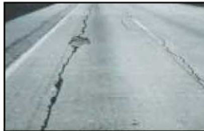
FIGURE 95 Distress Type CRCP 2—High Severity Longitudinal Cracking
