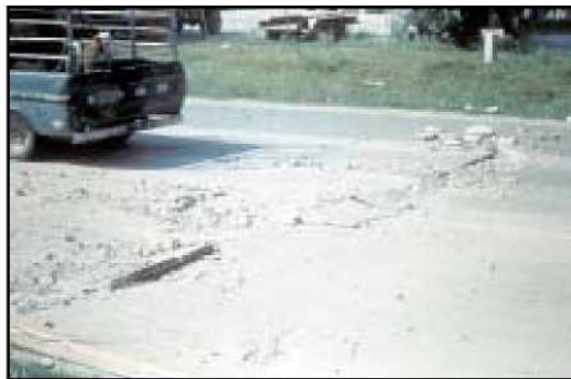
FIGURE 76 Distress Type JCP 11—A Blowup
