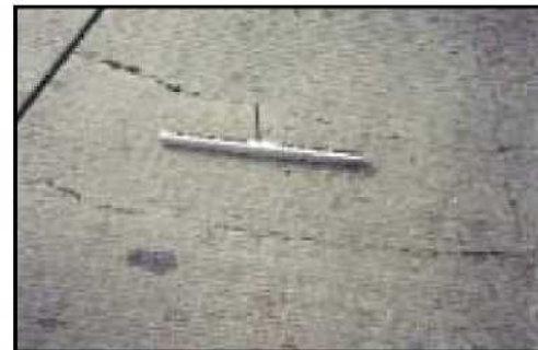
FIGURE 124 Distress Type CRCP 12—Low Severity Punchout
