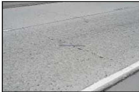
FIGURE 60 Distress Type JCP 4—High Severity Transverse Cracking
