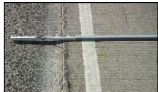
FIGURE 80 Distress Type JCP 13— Lane-to-Shoulder Dropoff
