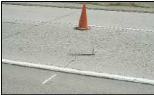
FIGURE 59 Distress Type JCP 4—Moderate Severity Transverse Cracking
