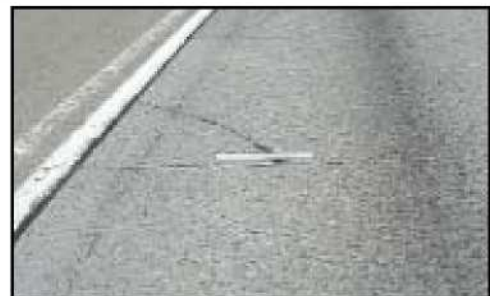
FIGURE 50 Distress Type JCP 1—Moderate Severity Corner Break
