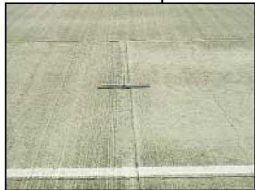
FIGURE 111 Distress Type CRCP 8—Low Severity Transverse Construction Joint Deterioration
