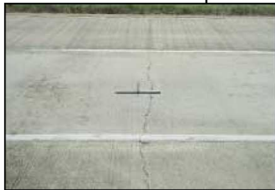
FIGURE 99 Distress Type CRCP 3—Moderate Severity Transverse Cracking
