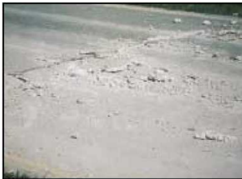
FIGURE 107 Distress Type CRCP 7—A Blowup
