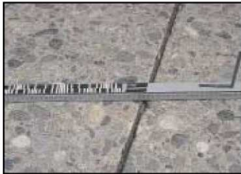
FIGURE 133 Distress Type CRCP 15—Longitudinal Joint Seal Damage
