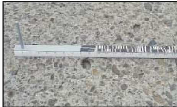
FIGURE 105 Distress Type CRCP 6—Popouts
