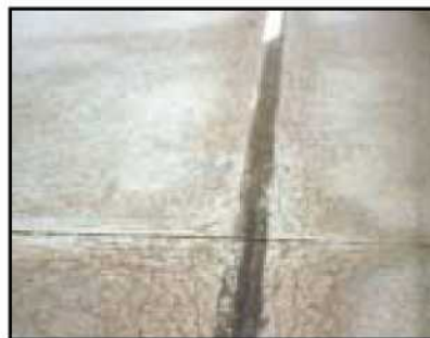
FIGURE 52 Distress Type JCP 2—Moderate Severity “D” Cracking with Well-Defined Pattern
