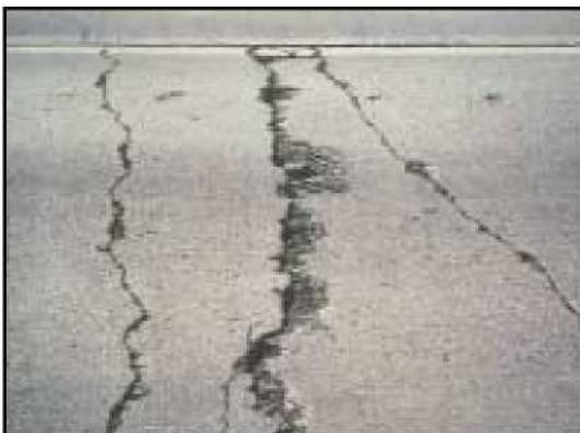
FIGURE 100 Distress Type CRCP 3—High Severity Transverse Cracking
