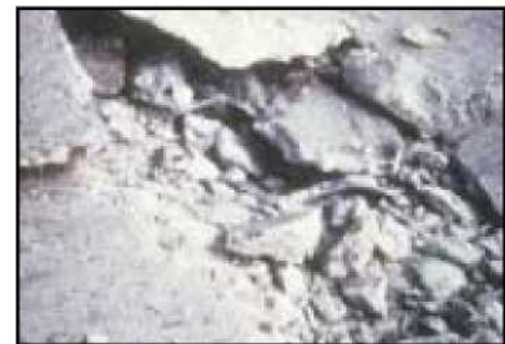
FIGURE 109 Distress Type CRCP 7—Exposed Steel in a Blowup
