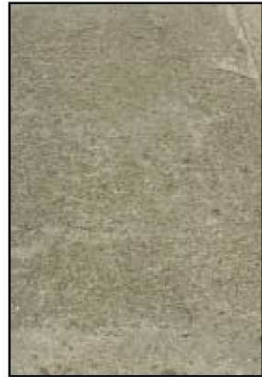
FIGURE 102 Distress Type CRCP 4b—Scaling
