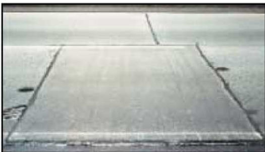
FIGURE 88 Distress Type JCP 15—Large, Low Severity Portland Cement Concrete Patch
