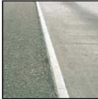
FIGURE 83 Distress Type JCP 14—Well-Sealed Lane-to-Shoulder Separation
