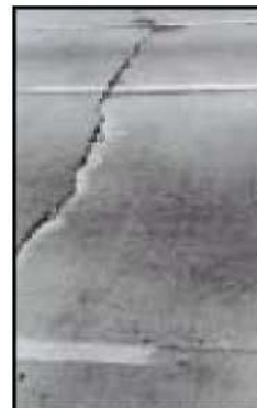
FIGURE 78 Distress Type JCP 12—Faulting of Transverse Cracks
