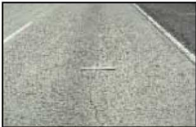
Figure 94 Distress Type CRCP 2—Low Severity Longitudinal Cracking
