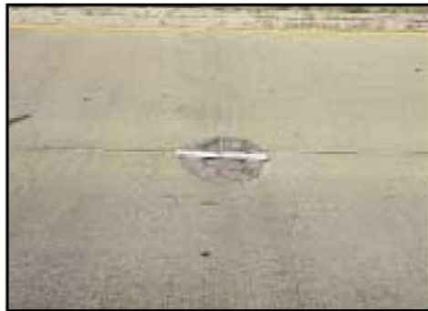
FIGURE 121 Distress Type CRCP 11—Moderate Severity Asphalt Concrete Patch
