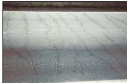
FIGURE 97 Distress Type CRCP 3—Transverse Cracking Pattern
