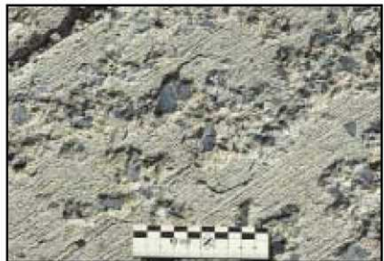
FIGURE 71 Distress Type JCP 8b—Scaling, Close-up View
