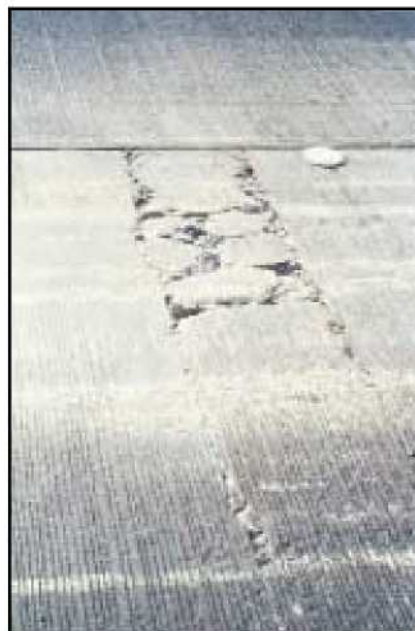
FIGURE 126 Distress Type CRCP 12—High Severity Punchout
