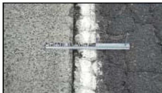
FIGURE 117 Distress Type CRCP 10—Close-up View of a Lane-to-Shoulder Separation
