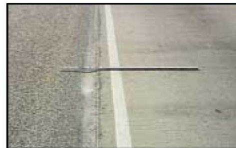
FIGURE 115 Distress Type CRCP 9—Lane-to-Shoulder Dropoff
