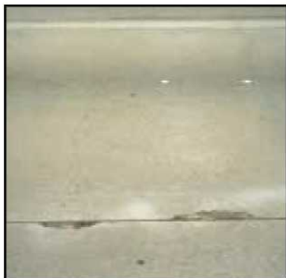
FIGURE 130 Distress Type CRCP 13—Moderate Severity Spalling of a Longitudinal Joint
