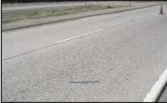
FIGURE 55 Distress Type JCP 3—Low Severity Longitudinal Cracking
