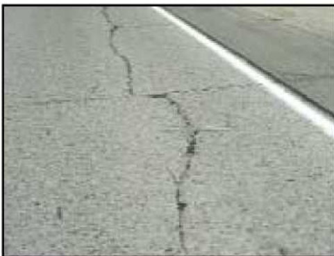
FIGURE 57 Distress Type JCP 3—High Severity Longitudinal Cracking
