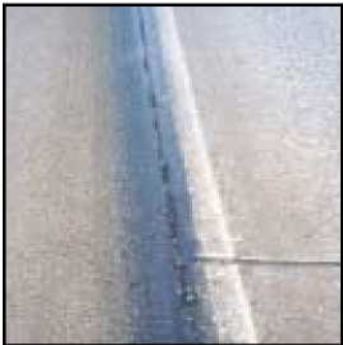
FIGURE 82 Distress Type JCP 14—Poorly Sealed Lane-to-Shoulder Separation
