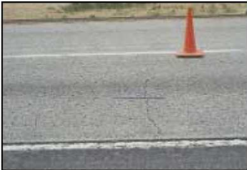
FIGURE 98 Distress Type CRCP 3—Low Severity Transverse Cracking
