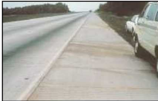
FIGURE 131 Distress Type CRCP 14—Water Bleeding and Pumping
