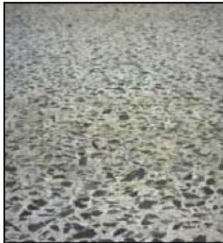
FIGURE 103 Distress Type CRCP 5—Polished Aggregate
