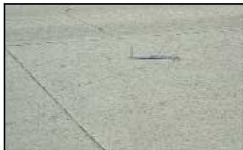
FIGURE 49 Distress Type JCP 1—Low Severity Corner Break
