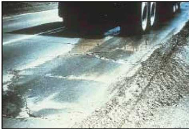
FIGURE 89 Distress Type JCP 16—Water Bleeding and Pumping
