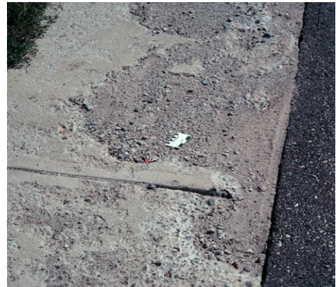
Figure 8.5-2 - A more severe example of scaling
