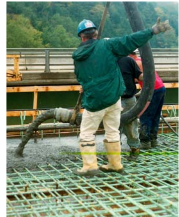
Figure 8.4.1-1 - Concrete being discharged into previously placed concrete to avoid segregation and damage to the epoxy coating.
