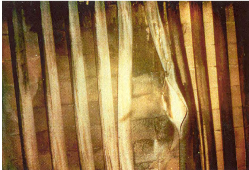
Figure 3-8. Failed Boiler Tube
