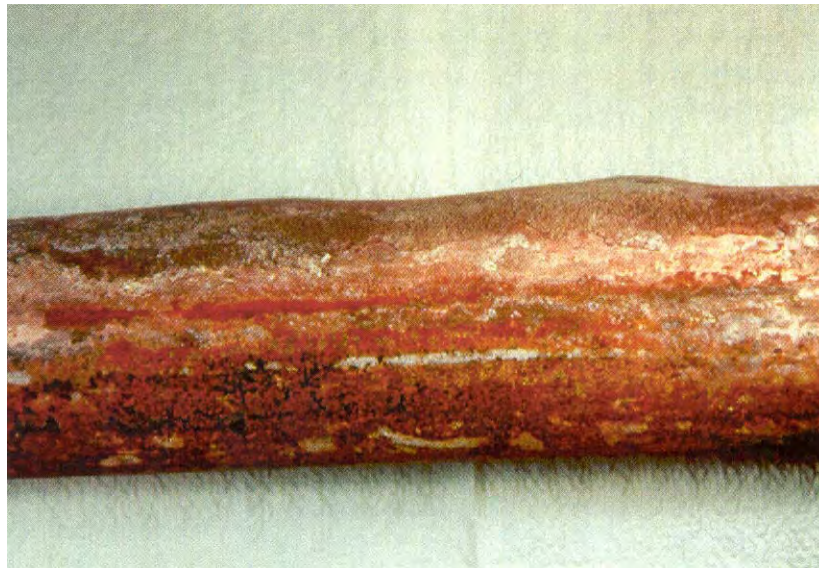
Figure 3-7. Metal Fatigue on Boiler Tube
