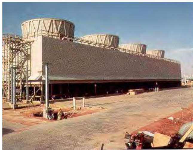
Figure 4-9. Counter-Flow Cooling Tower
