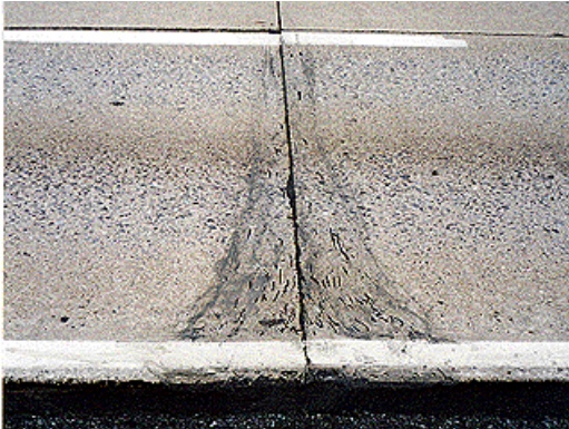
Figure 1-11 D-Cracking (Caltrans, 2004b)
