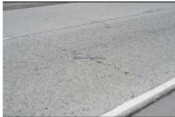
Figure 1-8 Transverse cracking (FHWA, 2003)
