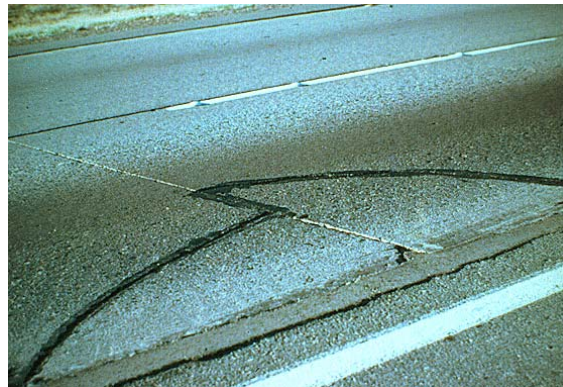
Figure 1-10 Corner break/cracking (Caltrans, 2004a)
