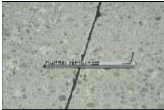
Figure 1-6 Example of joint seal damage (FHWA, 2003)
