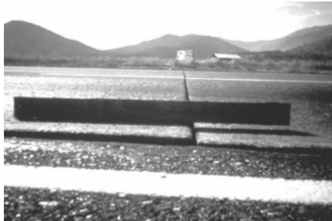
Figure 5-3 Faulting at a joint (FHWA, 2006)
