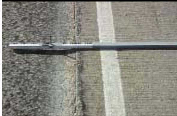
Figure 1-19 Lane/shoulder drop-off (FHWA, 2003)
