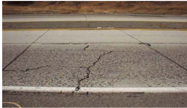
Figure 1-15 Severe surface abrasion with third stage cracking (Caltrans, 2004b)
