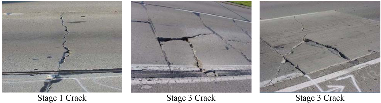
Figure 1-9 Examples of cracks at different stages (Caltrans, 2004a)
