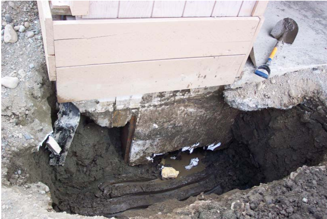
Figure 9: Foundation Condition after Subsurface Failure
