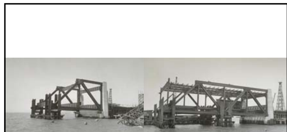
Deck Truss Span E-22 (near Oakland shore – Pier E-23 at right) Note the temporary truss support as it extends westward August 1934
