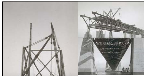
Left – traveler derrick Above – concrete (tower) pier supported deck truss spans – Oct./Nov. 1934
