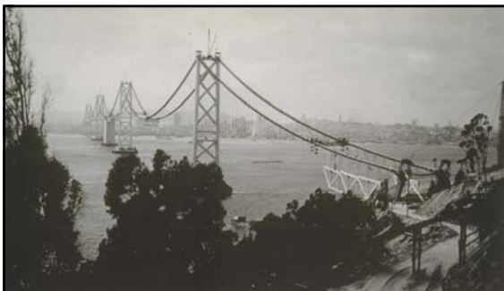
March 1936 Stiffening Truss section in place starting from mid-span between Tower Nos. 5 and 6. Truss sections being hung from Yerba Buena towards Tower No. 6 simultaneously
