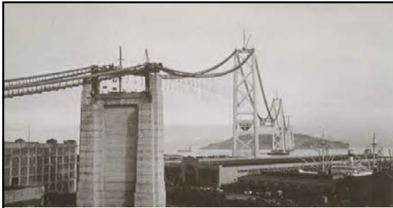
January 1936 Suspender ropes in-place. Barge at mid-span between Tower Nos. 2 and 3 with several stiffening truss section/s in-place. Hanging of the trusses began at mid-span rather than at the tower/s as would be typical for a suspension bridge). 337
