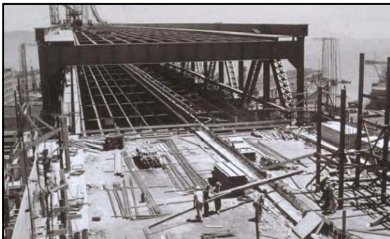
Atop San Francisco Anchorage (Viaduct Pier) (at interface with steel truss viaduct spans) June 1936
