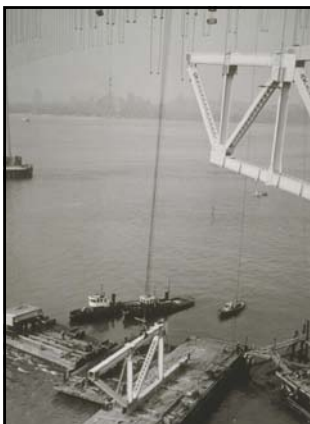
March 1936 A half-truss section is lifted off of a barge near Yerba Buena Island. Near the island, it was not feasible to lift full truss sections off barges as was the case in open water.
