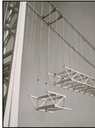
March 1936 Working from mid-span (between Tower Nos. 2 and 3), a stiffening truss section is lifted into place (near Tower No. 3). The special section/s adjoining the towers, W-4 and anchorages were left out until all other sections were in-place.
