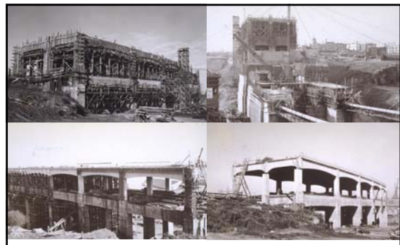
San Francisco Approach Viaduct November 1935 (upper left) / January 1936 (upper right) February 1936 (lower left & right)
