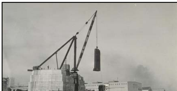
Tower No. 2 (atop Pier W-2) (stiff-leg derrick lifting pre-fabricated base cell section into position) March 1934
