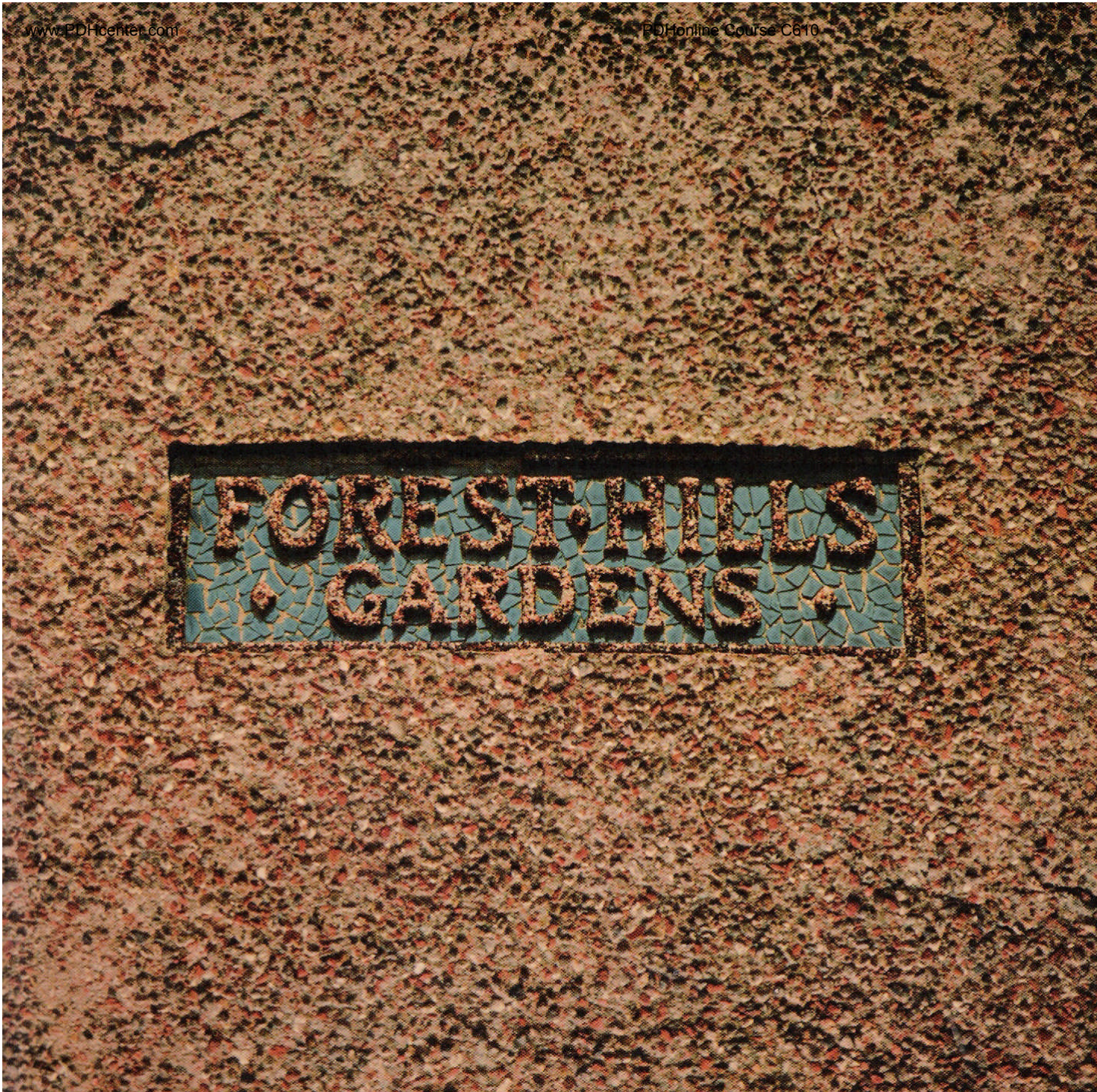
Close-up view of Pebbledash finish on face of balcony – FHG (LIRR) station (Station Square)
