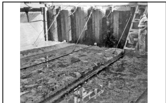
Cooling system pipes installed on top of five-foot pour (note horizontal construction joint-key construction joint-key; October 1933) 604
