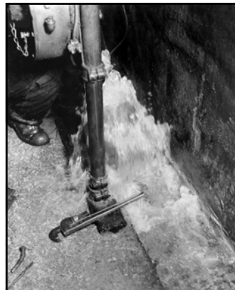
Close up of drain hole A-4, showing the water pressure present. Two hundred and thirty sacks of cement were injected into five drain holes to stop the leakage (June 1939).
