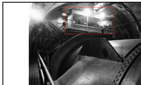
Scene in one of the original diversion tunnels at Hoover Dam showing a portion of one of the Penstocks which conveys water from Lake Mead to the Powerhouse. Each of the branch Penstocks was thirteen-feet in diameter. In the background (near the top of the Diversion Tunnel) can be seen the Visitor's Gallery , where the thousands who visit Hoover Dam annually can view the tunnel and Penstock.
