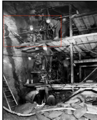
Drilling Jumbo in operation (on the right-side face of one of the Diversion Tunnels. When the drilling was complete, the holes were filled with dynamite, and the rock broken up by the explosions and removed. One-ton of dynamite was used for every fourteen-feet of tunnel dug (December 1931). 276
