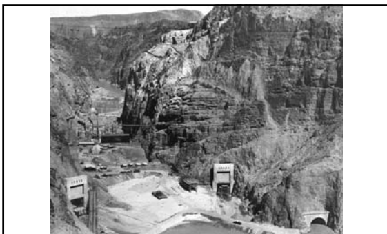
Looking upstream through Black Canyon (from permanent camera station). View shows dam structure and outlet portals of diversion tunnels Nos. 2, 3 and 4 (September 1933). 317
