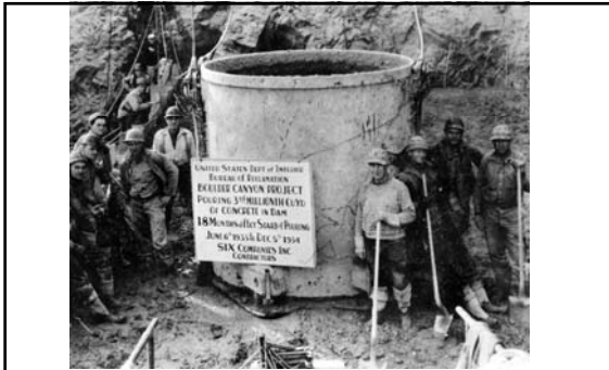
Placing the "third-millionth" cubic yard of concrete in Hoover Dam; December 5 th 1934 667
