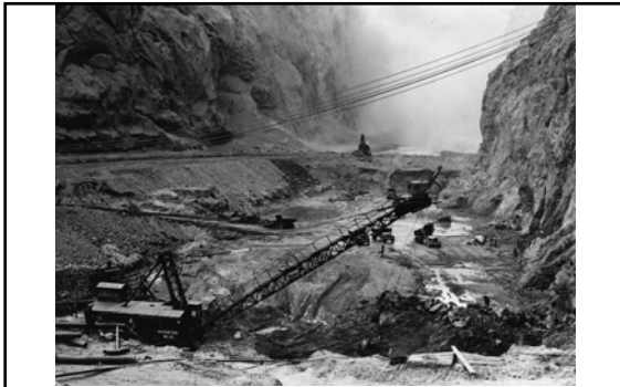
Looking downstream into the Upper Cofferdam excavation (dyke and restricted river channel are at left; October 1932)
