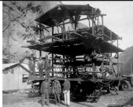
View of drilling Jumbo taken outside the Diversion Tunnels. It was welded steel construction, mounted on a truck chassis (December 1931). 274
