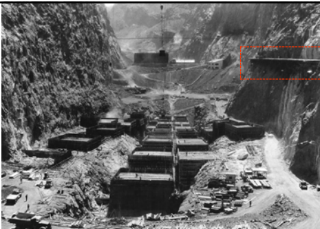
Looking downstream across dam construction (from upstream cofferdam). Trestle over which electric trains operated can be seen against the canyon wall (at right; July 1933). 635
