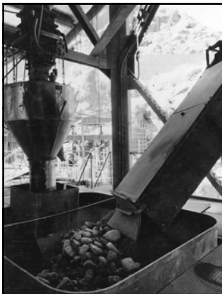
Aggregate delivery into mixer hopper at Six Companies' High-Level concrete mixing plant, (cement batcher and delivery seen at left; April 1933)
