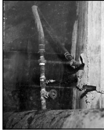
Detail showing connection from header pipe to circulating system in the dam's pre-cooling system (February 1934)
