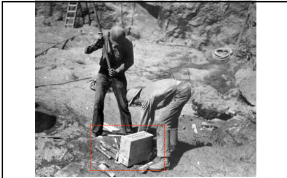
Workmen loading hole with dynamite preparatory to blasting (in the Nevada power plant site; March 1934)
