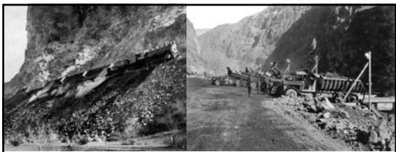
Left: "Muck Train" dumping along the railroad right-of-way, upstream from the river camp (showing western side-dump/drop-door type of cars; January 1932) Right: trucks (hauling spoil from Diversion Tunnel inlet headings) dumping their loads into railroad cars at transfer dock operated by Six Companies (near low level concrete mixing plant in Black Canyon; February 1932) 477
