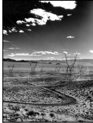
Hoover Dam transmission towers passing through the desert
