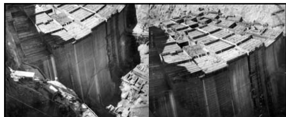
Upstream face of dam structure (as seen from cableway skip operating between Intake Towers). Top forms at Elevation 810 (March 1934).
