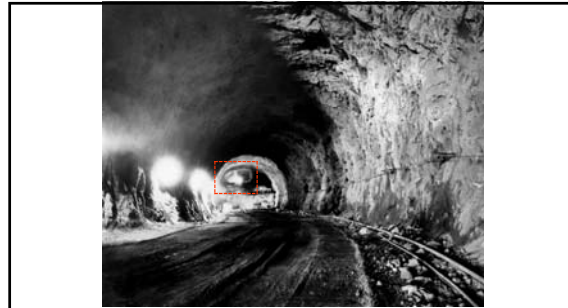
Interior of one of the Diversion Tunnels. The Drilling Jumbo is working at the tunnel face (the twelve-foot by twelve-foot top-heading can be plainly seen; January 1932). Each tunnel was dug to a diameter of fifty-six feet. With the addition of the three-foot thick concrete lining, the finish diameter of each tunnel was fifty-feet. 476
