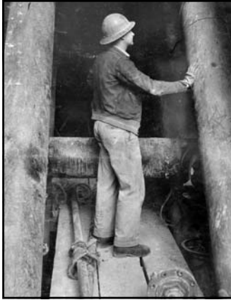
Photo showing installation of pre-cooling header pipes in eight-foot wide slot through middle of dam (both the lead and return pipes are shown). Over 582 miles of cooling pipes were placed within the concrete of Hoover Dam (February 1934).
