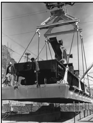
Railroad car (gondola), containing lower bearing support bracket for N8 generator, being transported by the 150-ton cableway preparatory to lowering to power plant (January 1961)
