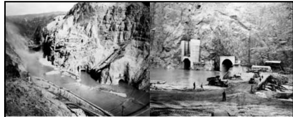
Left: Lower Portals of Diversion Tunnels Nos. 3 and 4 (after diversion of the Colorado River was completed; November 14 th 1932)
