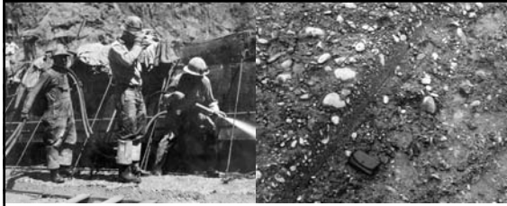
Left: washing surface concrete in dam pour using compressed air and water Right: top surface of test pour in Column H-5 at Elevation 635. Photo was made twelve hours after pour was finished and after surface was given its first washing (September 1933).
