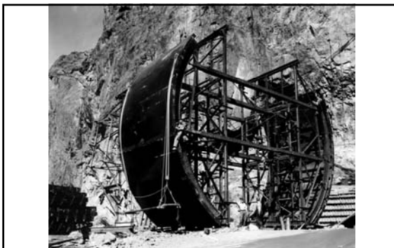
A close-up view of a section of the forms used in placing the side-wall sections of the concrete lining in the Diversion Tunnels (Aug. 1932) 483
