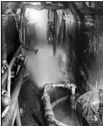
The quantity of water (entering the 553 gallery) exceeded the capacity of the temporary pumps. The excess was collected and delivered to the 647 gallery (June 1939)
