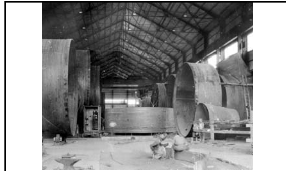
View looking (longitudinally) through the Babcock & Wilcox Co. plant showing the fabrication of thirty-foot diameter steel Penstock sections; August 1934
