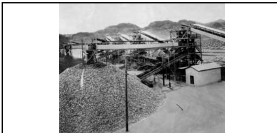
Gravel screening plant (view from the crusher bin; April 1932). Live storage of aggregates on the left, screening towers on the right. At the screening plant, four screening towers separated the aggregate into different sizes: fine , intermediate and coarse gravels, and cobbles (three-inches to nine-inches in diameter). Anything over nine-inches was run through a crusher and screened again. The separated gravel and cobbles were transported to the mixing plants by train. 575
