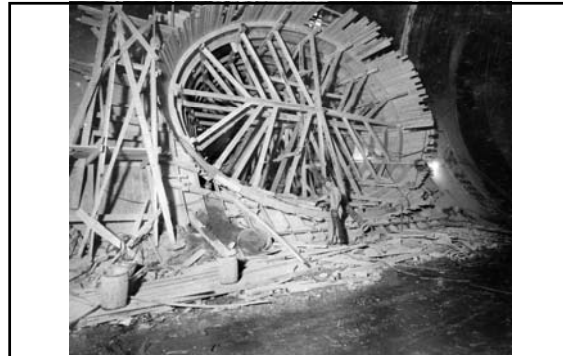
Timber formwork for intersection transition between Diversion Tunnel No. 3 and Penstock tunnel (June 1934)
