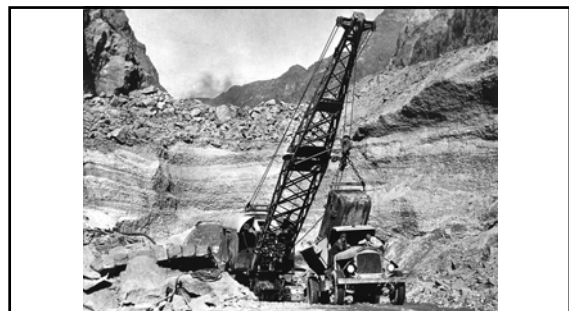
Looking upstream through Black Canyon toward the dam site (showing condition after the diversion of the Colorado River). Lower levels of canyon choked with material blasted and scaled from the canyon walls. A downstream rock barrier can be seen in foreground (January 1933).
