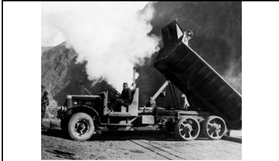
A ten cubic yard Moreland truck dumping directly in the side-dump railroad cars at the dump hopper (in front of the low level mixing plant). Truck was carrying muck from upper portals of the Diversion Tunnels (January 1932). 247
