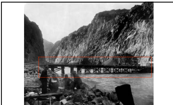
Prior to the completion of the steel suspension bridge, a temporary pile and trestle bridge was erected to enable the removal of excavated rock from the upper portals of the Arizona diversion tunnels. 141
