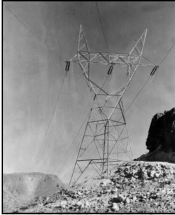
One of many transmission towers comprising the City of Los Angeles' 287,500 volt transmission line
