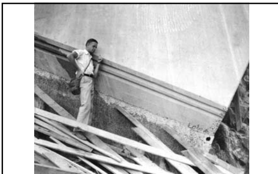
Construction joint (at base of side-wall) along vertical curve transition into inclined Spillway tunnel (Nevada Spillway; September 1933) 621
