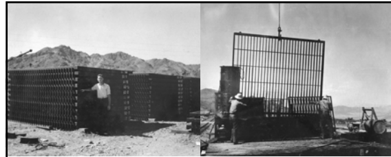
Left: Intake Tower Trashrack steel stock-piled in Boulder City storage yards prior to coating (May 1935) Right: Intake Tower Trashrack steel being given final pitch coat (unit has already received primer coat; June 1935)
