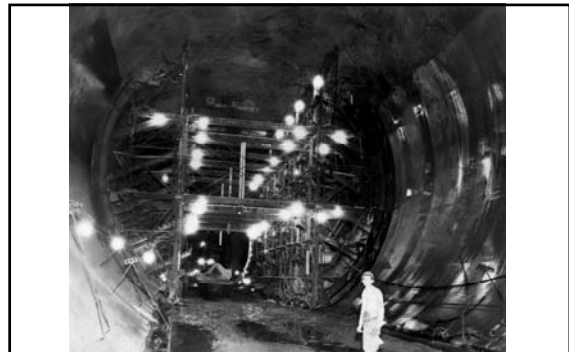
Showing the method of construction and operations of the Side-Wall Jumbo for placing the lining in the Diversion Tunnels (June 1932)
