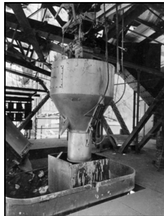
Cement batcher assembly over aggregate hopper at the Six Companies' High-Level concrete mixing plant (feed mechanism and lever arm connection to scales seen at top; April 1933)
