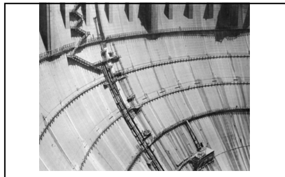
Upper section of downstream face of dam showing catwalks and grout distribution pipes installed. Elevation 1025 and 1075 grout lines are seen between two construction catwalks (April 1935). 622
