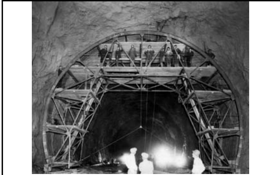
Close-up showing details of Trimming Jumbo used in scaling walls of diversion tunnels and removing projecting rock (April 1932)
