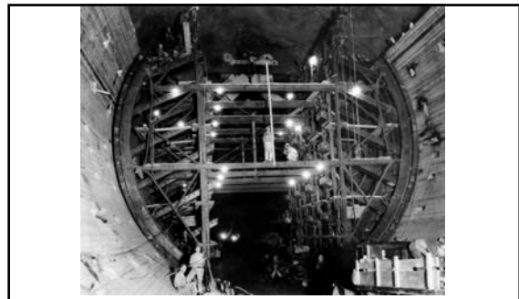
The Diversion Tunnels were lined with concrete and made to conform to an exact fifty-foot circular section by means of temporary wooden panel forms (July 1932)
