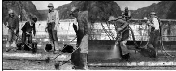
Left: brushing top of concrete to remove laitance preparatory to pouring next higher lift (January 1934) Right: cleaning top of concrete with water under air pressure preparatory to placing next pour (January 1934)
