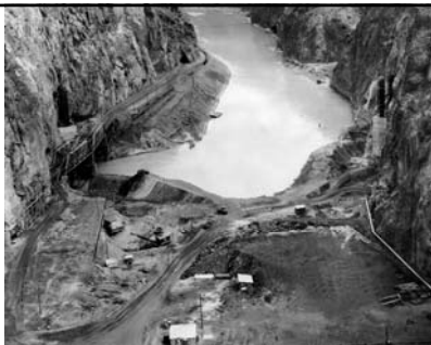
Upper portals of the Diversion Tunnels. The dyke being built is at Elevation 690 (which is the elevation of the top of the tunnels). The upstream dyke required 732K cubic yards of concrete and the downstream dyke required 500K cubic yards (November 1933).
