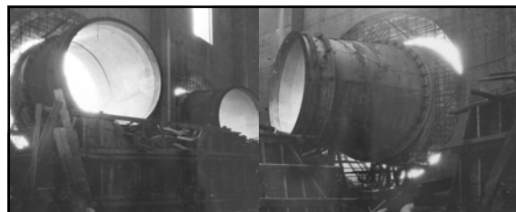
Left: portion of front wall of Nevada canyon wall Outlet Works structure showing discharge guide tubes for 84-inch balanced needle valves (July 1935) Right: discharge guide tube for 84-inch balanced needle valve (July 1935) 726
