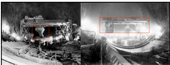
Left: concrete lining in Diversion Tunnel No. 2. Two cubic yard buckets were suspended from the gantry crane (March 1932). Right: dumping concrete from buckets suspended from gantry crane into invert forms in Diversion Tunnel No 2. Screed is seen below crane, finishing platform is seen in front of the screed (April 1932). 479
