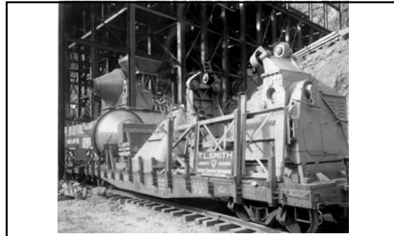
Mixers being unloaded from railroad cars. These mixers were four cubic yards capacity and had a cycle of three-and-a-half minutes for loading, mixing, and discharging (January 1932).
