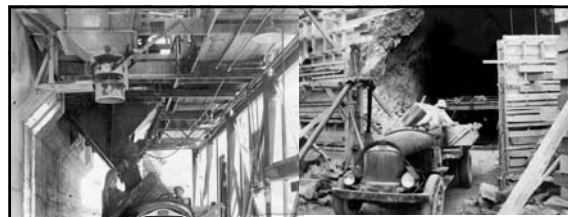
Left: loading concrete into two cubic yard bottom dump buckets at Six Companies' low level concrete mixing plant. Buckets were hauled (two to a truck) into Diversion Tunnels where they were handled by crane into position over invert forms (April 1932) Above: truck loaded with concrete entering the upper portal of Diversion Tunnel No. 2 (through opening left in Cofferdam; April 1932) 478
