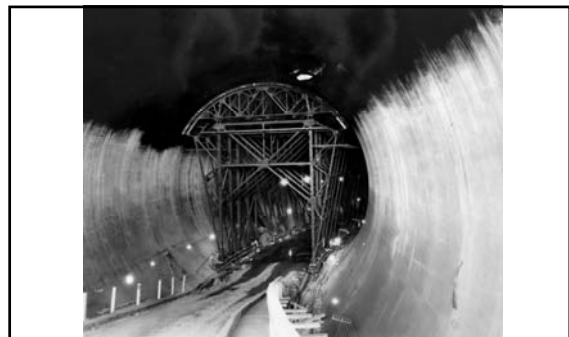
Interior of Diversion Tunnel No. 4 (near the upper portal) showing the Arch Jumbo in place. The arch section has been coated with a bituminous surface for curing the concrete (June 1932).
