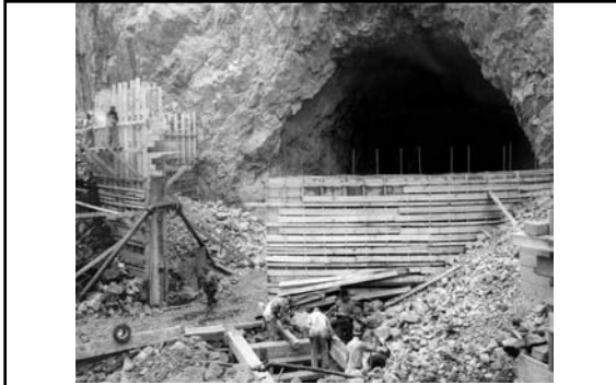
Semi-circular (arch) concrete Cofferdams being erected around the portal of Diversion Tunnel (as protection against high water; April 1932) 523
