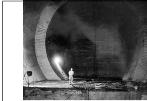
Upstream tunnel plug construction in Diversion Tunnel No. 3. This view shows the downstream face of the completed section of the plug with the lower pours of the next lift in place (June 1934) 536
