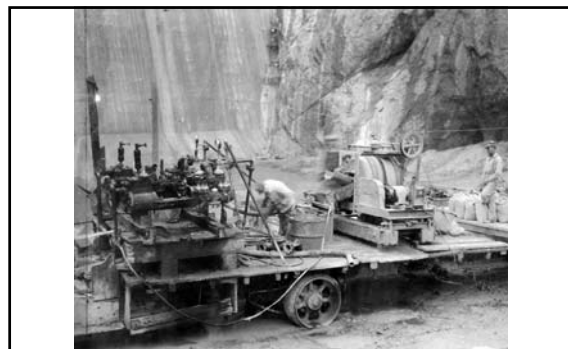
Grout Rig on upstream face of dam. This rig is forcing grout into holes in the Nevada abutment (December 1934). 624
