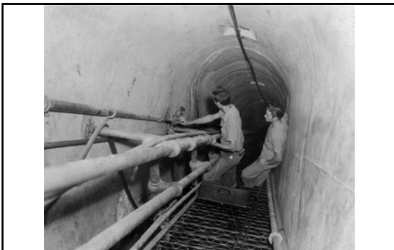
The grout was pumped through pipes through the Inspection Galleries deep into the dam (October 1940)
