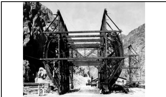
Fabricated steel forms for placing the three-foot thick lining in the side-wall section of the Diversion Tunnels being erected outside the upper portal of Diversion Tunnel No. 1 (July 1932)
