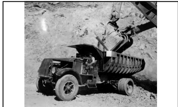
Mack truck with fourteen cubic yard body being loaded at the Nevada Spillway cut. Five similar trucks were being used on this operation (March 1932). 250
