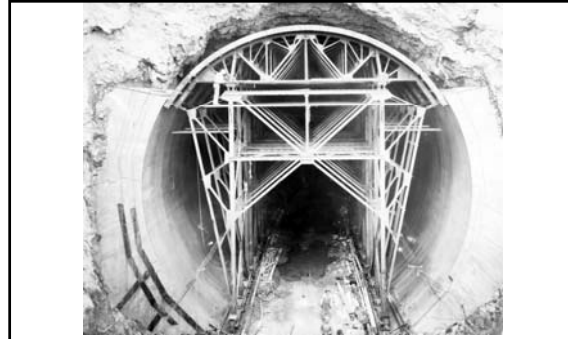
Placing steel form for the first pouring of concrete in the lining of the arch section of the Diversion Tunnels. View shows upper portal of Diversion Tunnel No. 4 (June 1932). 482
