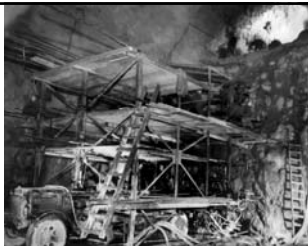
View of a drilling Jumbo tacked up to the tunnel-face (showing the method of construction and mounting; December 1931). The jumbo was backed up to the working face and 24 to 30 drills went to work, drilling powder holes into the rock. A drilling jumbo allowed half of the tunnel face to be worked on (with all the holes being drilled simultaneously). When the holes in that section were finished, the jumbo moved to the other side of the rock-face and began drilling, while the finished holes were packed with powder and wired. When both sides were drilled, the jumbo was removed. Eight of these jumbos were constructed enabling the drilling and blasting to be accomplished in record time. 275
