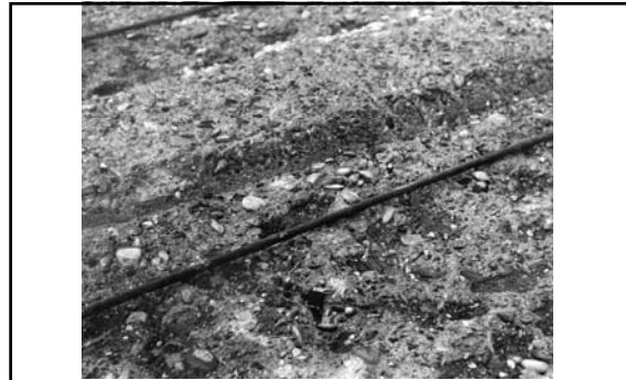
Detail of construction joint cleanup showing cooling system pipes and horizontal construction joint keys (test pour in Column H-5, Elevation 630; August 1933) 620
