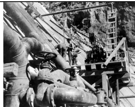
Booster pump and pipe connection into dam cooling system (at Elevation 795; April 1934)
