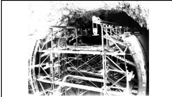
Detail picture of the Side-Wall Jumbo used in placing the three-foot thick lining in the Diversion Tunnels. The side winds were jacked into place, and concrete was poured through ports by means of a traveling crane and two cubic yard buckets (April 1932). 481
