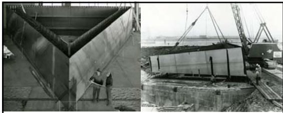
"...The Arch is being built in sections. 'Sandwich' walls are shipped to St. Louis from Pittsburgh, where they are fabricated, and are put together on the site to form triangular sections about twelve feet high. These sections, weighing up to 50 tons, are hoisted into place by a derrick..." The Rotarian, June 1963
