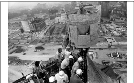
Placing concrete between inner and outer steel skins (below the 300-foot level)
