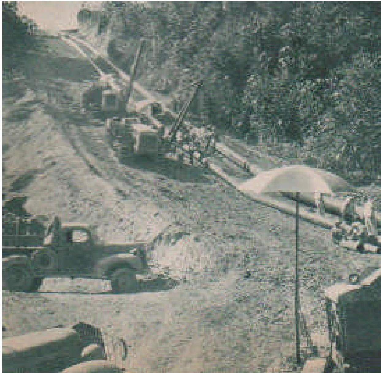
Left: caption: “Building the $20,000,000 Panama fuel pipe line with a daily capacity of 265,000 barrels of fuel oil – a wartime project”
