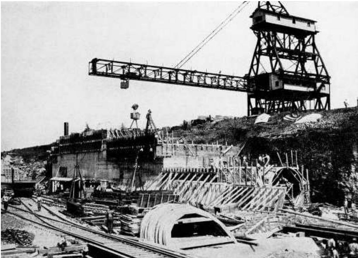
Top L&R : caption: “Steel Forms, Gatun Locks” Left : caption: “Traveling Crane Handling Concrete in Lock Building.’ These cranes are the striking feature of the Canal landscape, handling thousands of tons of concrete daily.”
