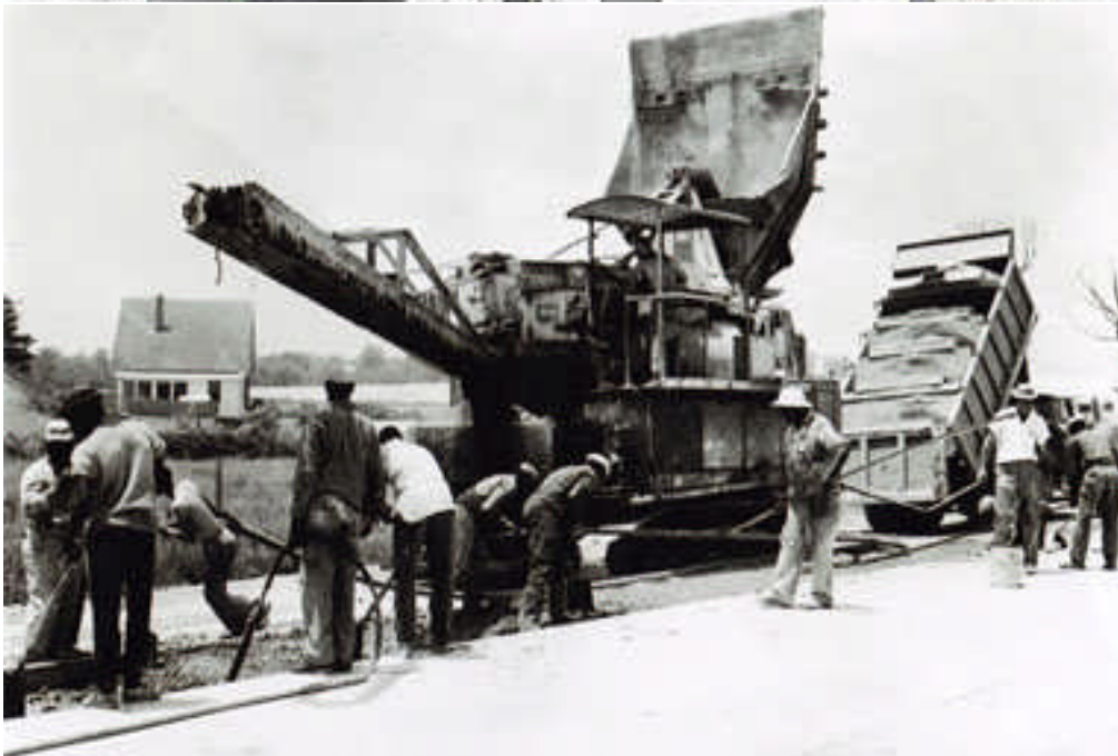
Above L&R: caption: “Virginia Bridge construction I-64 - in Chesapeake County, south of US 460 & S.R.166”
