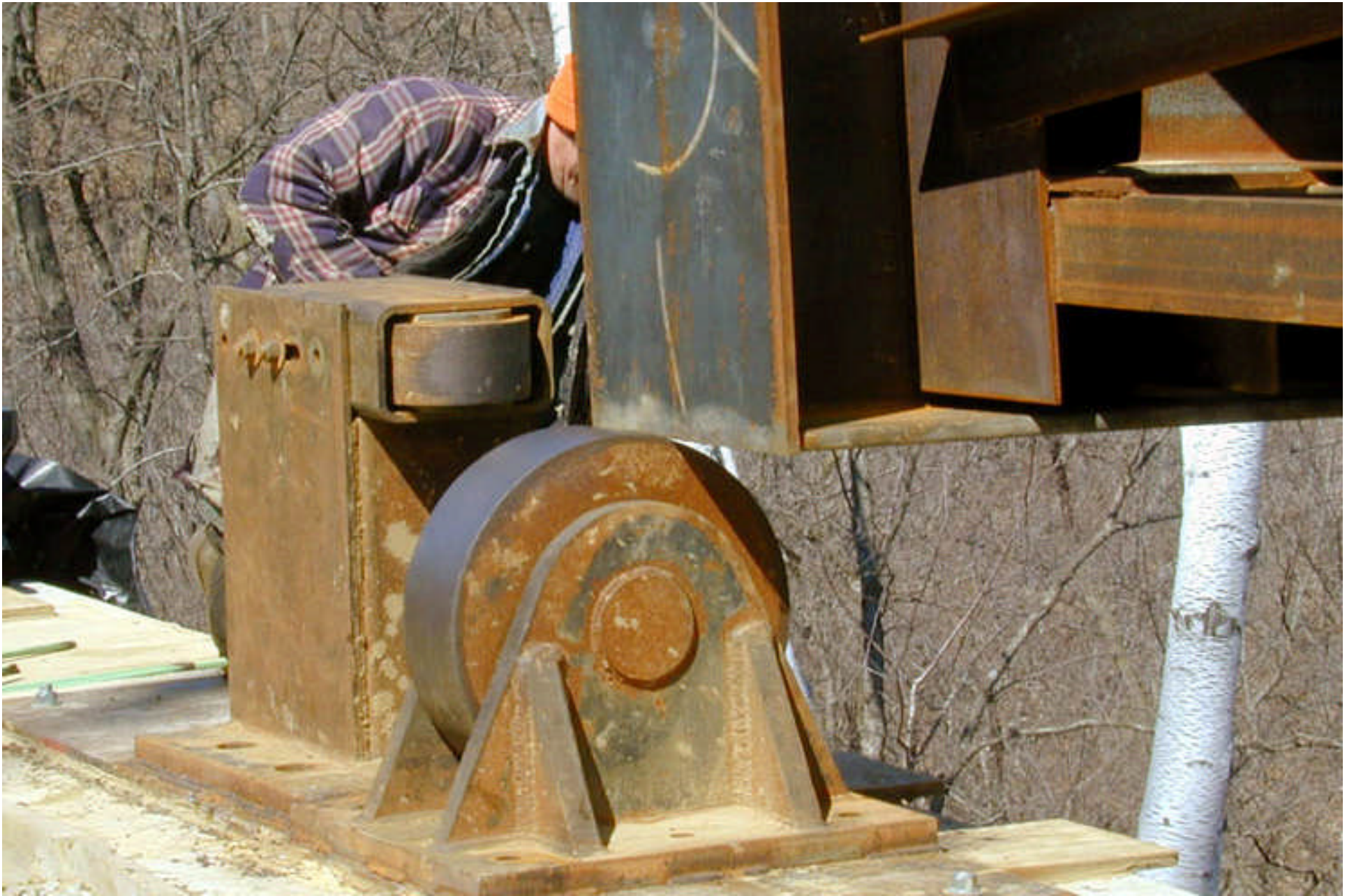
Above: caption: “Tip of launching nose landing on roller used during the bridge launching”
