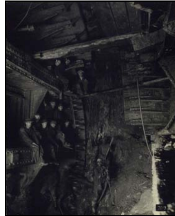
Left: caption: "North Tunnel - New York and New Jersey shields the day prior to their junction"
