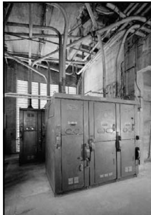
Left: caption: "New York Land Ventilation Building, 4th Floor, Detail Showing Main Feeder Station"
