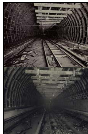
Top: caption: "Concrete Roadway. Beginning of sidewalk, and reinforcing of sidewalk, North Tunnel. View shows construction track on roadway and roof rebolting and caulking platform."
