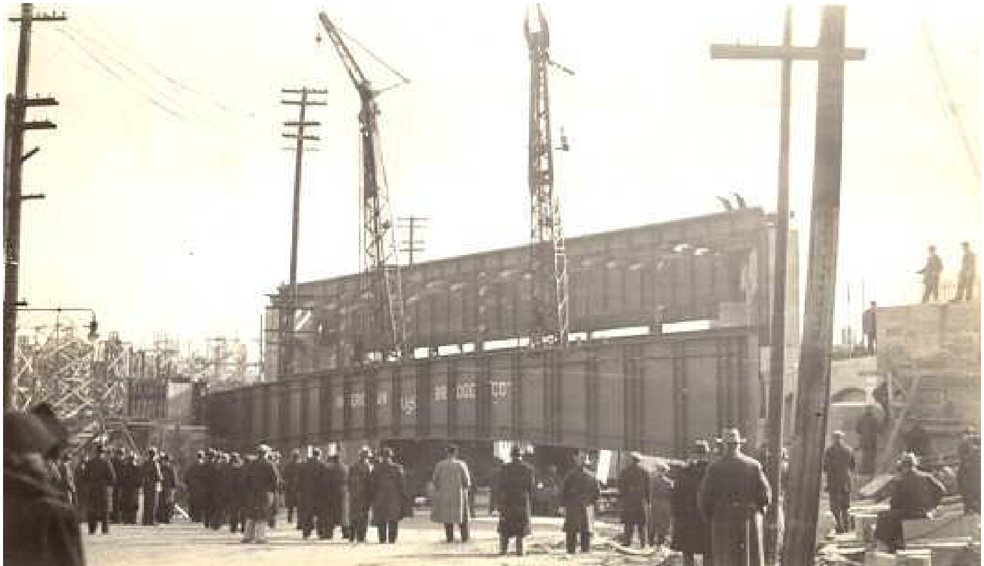
Above: caption: “Installation of the bridge carrying the Lincoln Tunnel approach over Park Avenue. Placing 55-ton steel to complete the ramp on Park Av.”
