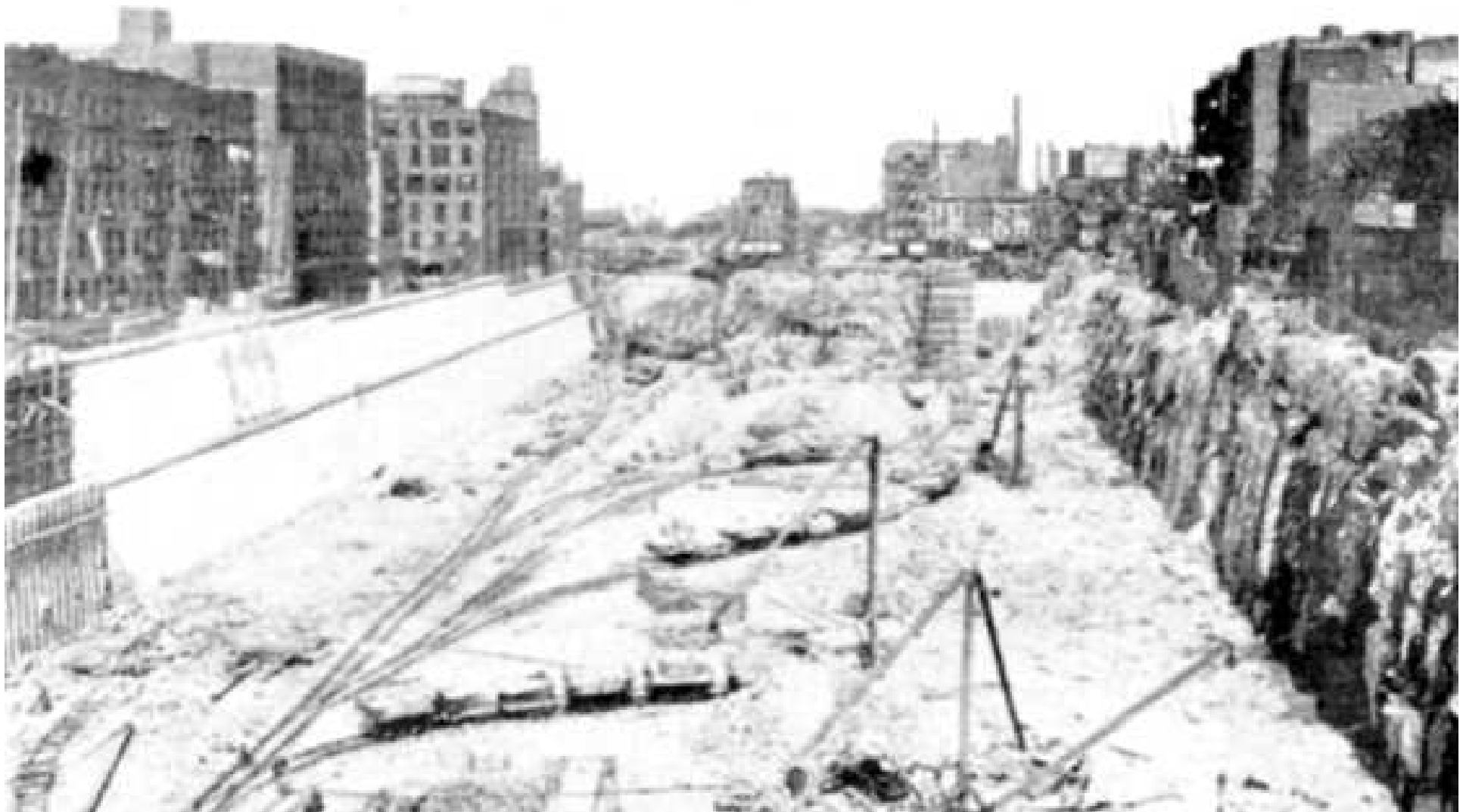
Above: caption: “View looking West from Ninth Avenue Elevated Railway, showing condition of Work.” Note retaining/face wall at left is nearly complete while the wall at right is still exposed.
