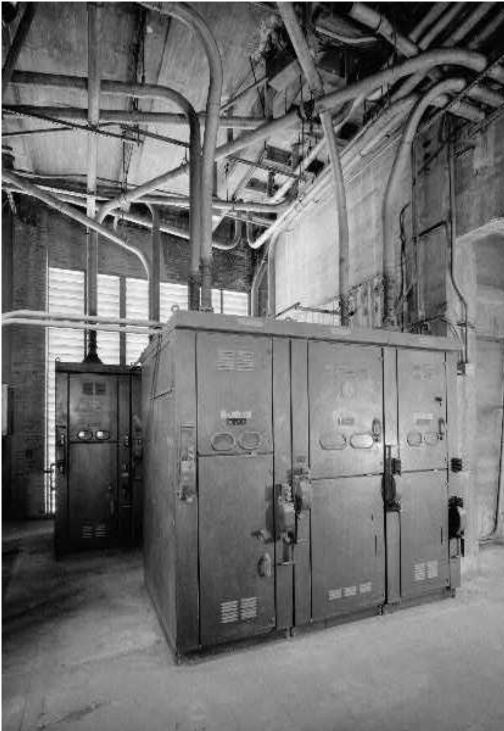
Left: caption: “New York Land Ventilation Building, 4th Floor, Detail Showing Main Feeder Station”
