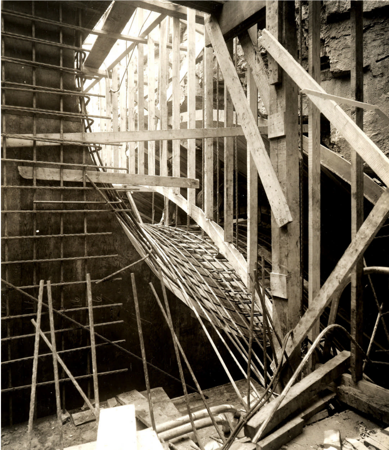
Left: caption: “Forms and Reinforcing for Air Ducts and Ventilation Shaft, Weehawken, New Jersey”
