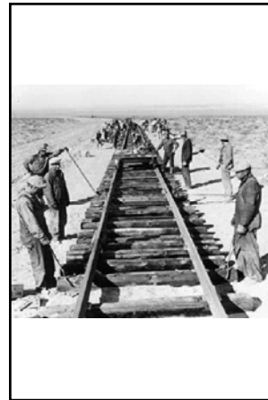
"They could lay from one to three miles of track per day as they had material"
