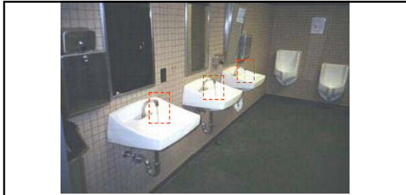
Above: the extremely economical "push-rod" automatic faucet controls (highlighted) reduced water consumption by over 40% and minimized piping redundancies by mixing hot and cold water into single pipe supply lines. Thus, a single automatic mixing valve (for a gang of lavatories) allowed just a single supply line to each, saving on installation and maintenance expense. Water conservation measures for the one-hundred and twenty-five building occupants also included the use of water-less urinals. 55
