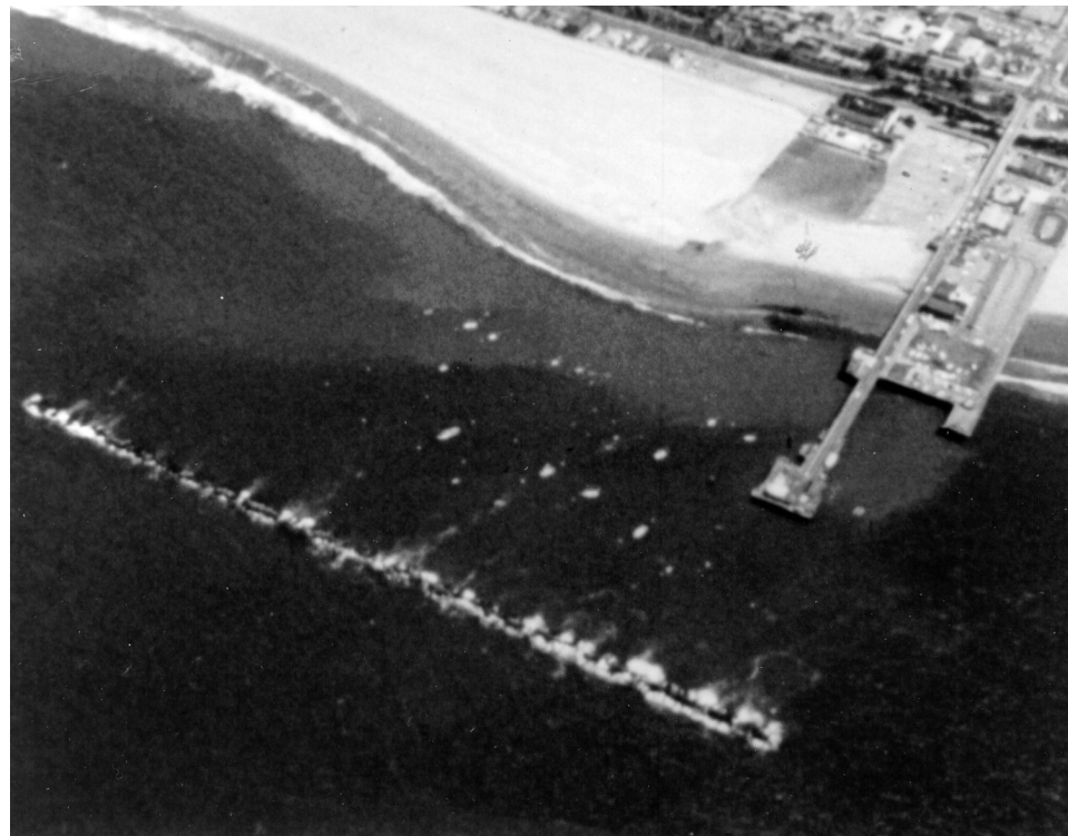
b. Deteriorated breakwater allowing wave transmission
