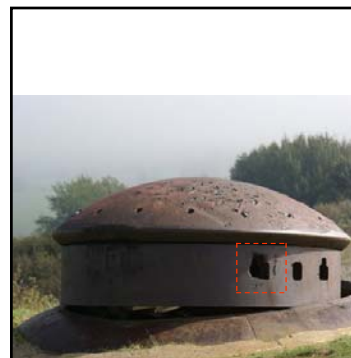
Left: this 75mm AM turret was equipped with mixed weapons. The preliminary bombardment of Petit Ouvrage La Ferte had disabled the turret, sticking it in the up position, making it unable to turn (traverse). A German shaped charge opened a hole in the weapons embrasure (left). The Germans then dropped a charge into the turret itself. The resulting explosion blew the turret into the air, and it dropped down, falling off center.
