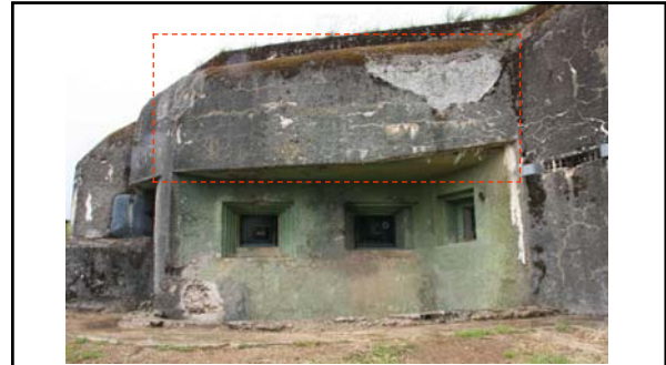
CORF interval casemates had their main embrasures protected from plunging artillery fire by a roof overhang Above: caption: "The overhang as can be seen at Block 1 of PO La Ferte. The grey square in the concrete at the left is the armored door of a searchlight. This is a typical construction for casemates/ouvrages built after 1935. Original camouflage paint can be seen around the embrasures."
