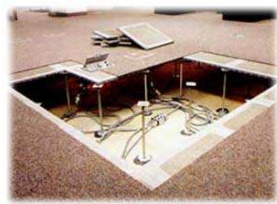
Figure 2-7 : Typical Raised Floor
