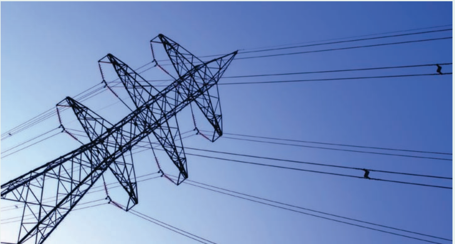
Transmission of new power can often be a challenge, but fortunately, a 138-kVA transmission line with plenty of spare capacity was available to U.S. Geothermal along the northern boundary of the Raft River geothermal field.
