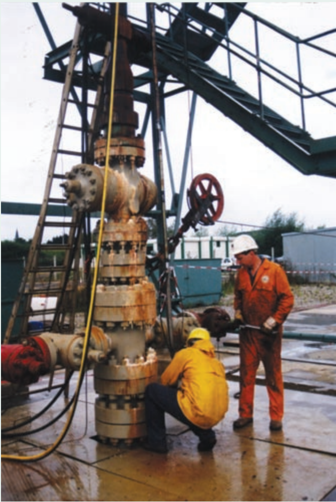
Flow testing is among the field tests being performed in Soultz, France, in an attempt to better understand EGS potential.
