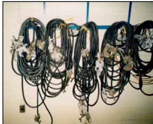
Figure 24. – Example of proper storage of protective grounds, coiled and hung on wall.
