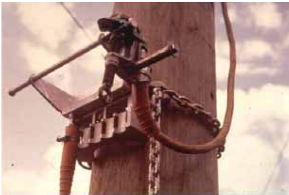
Figure 20. – Example ground cluster bar attached to wood pole. The bar provides convenient point of attachment for protective grounds and a bond to the pole structure ground wire, if provided.
