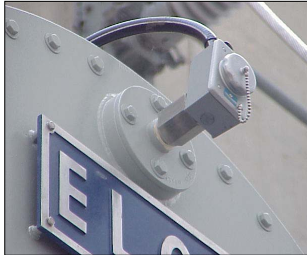
Figure 13.—Bladder Failure Relay.
