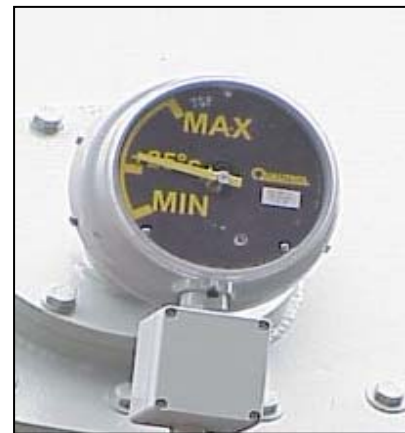
Figure 8.—Conservator Oil Level.
