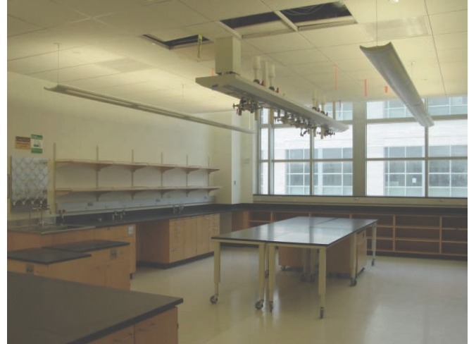
Figure 5: Aisle-mounted indirect luminaires suspended in relation to the overhead service trunk can maintain good-quality lighting regardless of the position of the movable benches, as long as the ceiling remains somewhat consistent.
