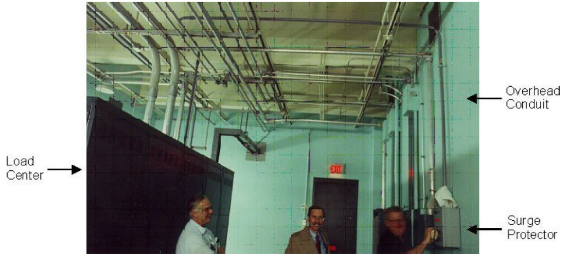
Figure 4. Unacceptable Installation with Long Surge Protector Leads
