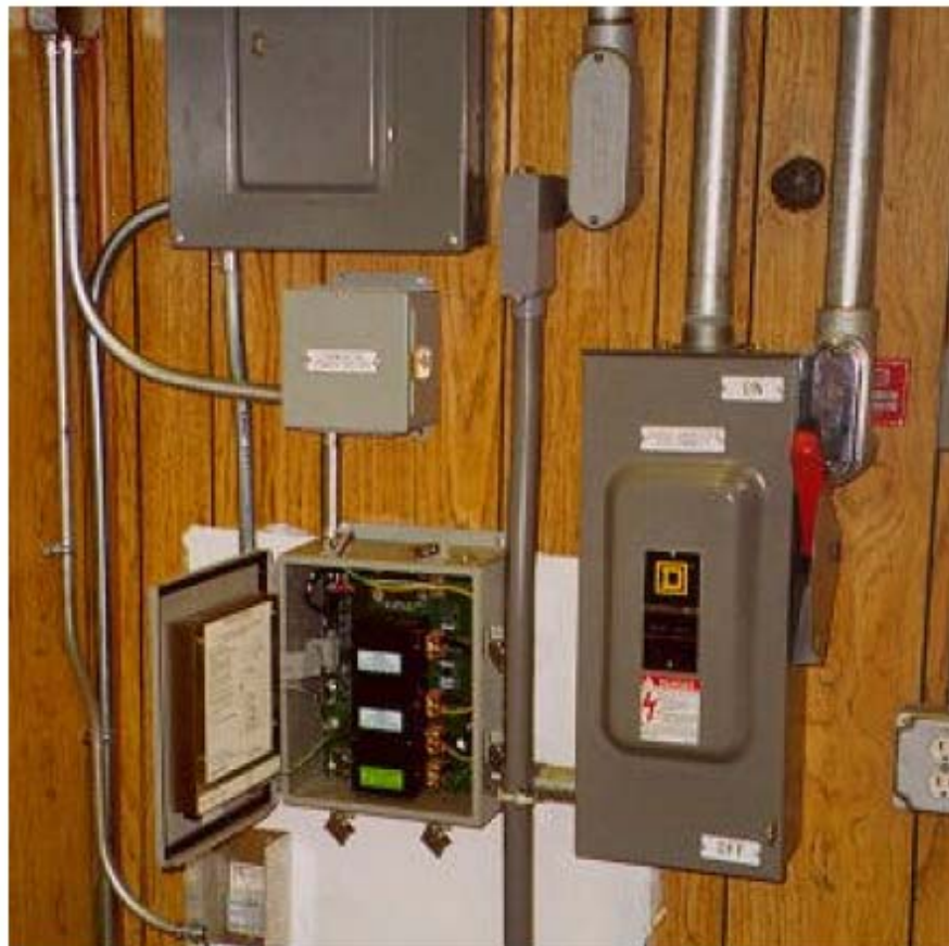
Figure 5. Less-Than-Optimal Installation by Including Safety Switch
