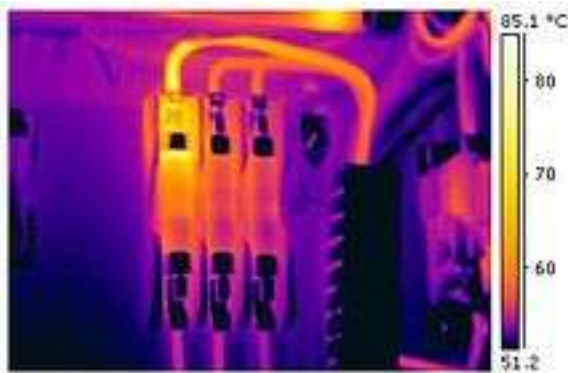
This thermogram shows a fault with an industrial electrical fuse block.
