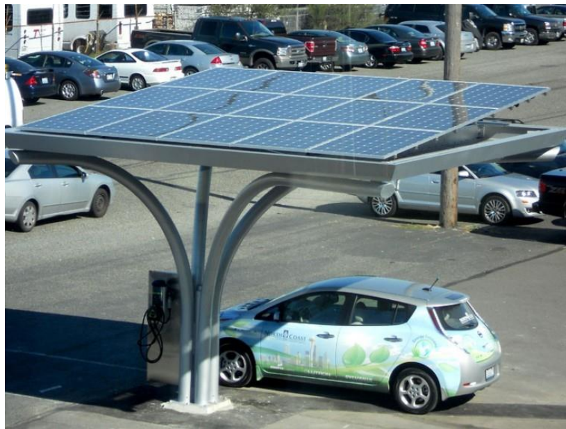
Solar Charge Station
