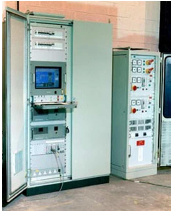
Figure 22: Master Control Station
