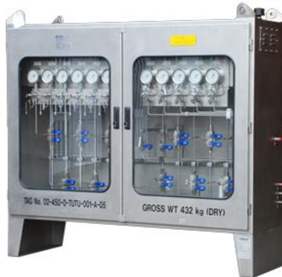
Figure 23: Topside Umbilical Termination Assembly (TUTA)
