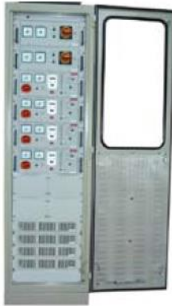
Figure 24: Electrical Power Unit
