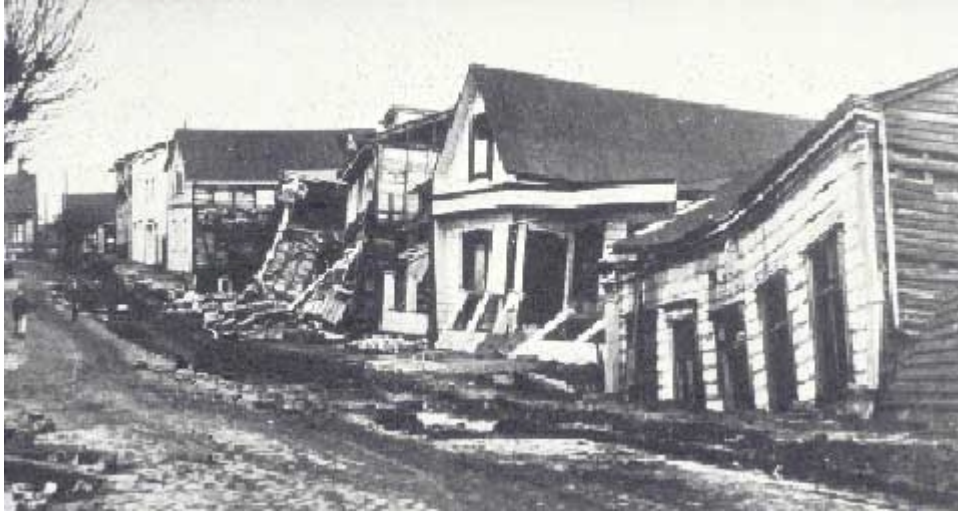
Figure 9: Valdivia suffered severe damage because of its proximity to the epicenter of the May 22, 1960 earthquake.
