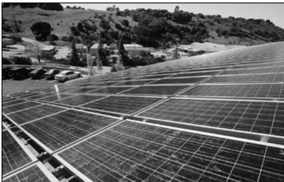
This installation of PV panels, equivalent to one-half of an acre, covers the roof of the new San Mateo County Forensics Laboratory.
