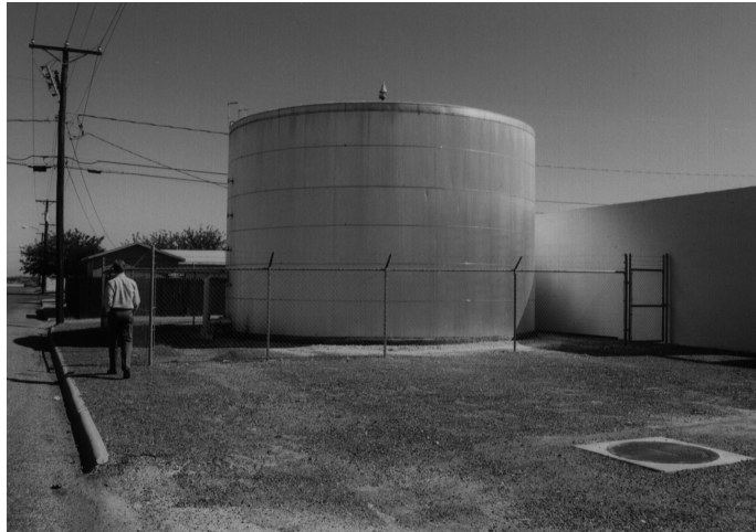
Figure 8-2. Chilled Water Storage Tank at the Hospital in Monahans, Texas
