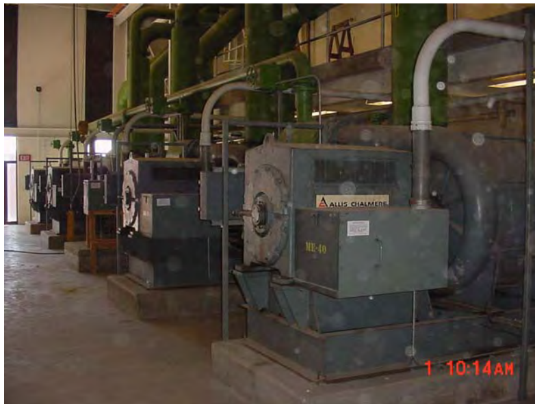
Figure 3: Multi-stage Centrifugal Blowers - GBMSD - De Pere Wastewater Treatment Facility (Photo provided courtesy of the Green Bay Metropolitan Sewerage District)
