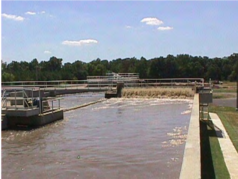
Figure 2: Oxidation Ditch/Aeration Rotor at the City of Bartlett WWTP #1 (Photo provided courtesy of the City of Bartlett Wastewater Division)
