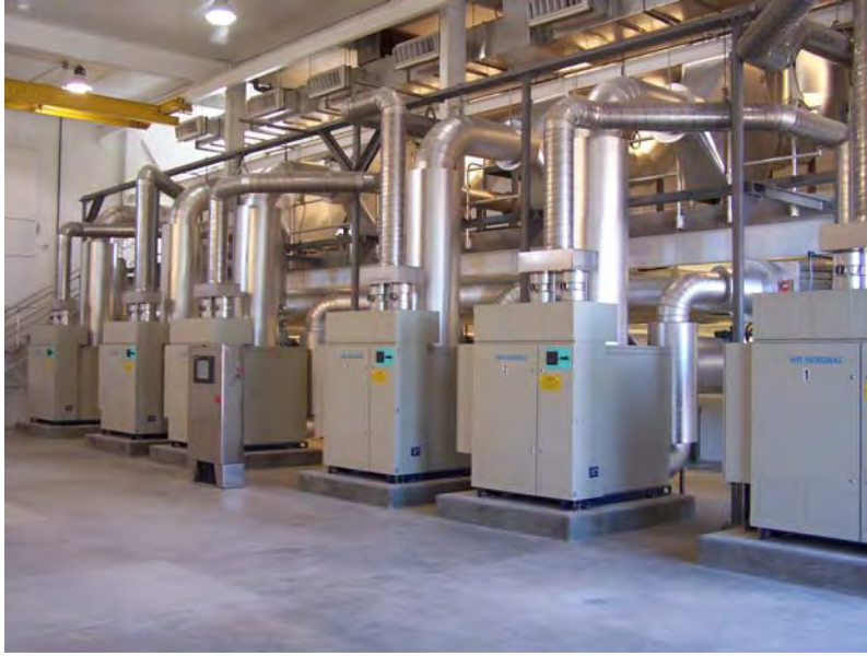
Figure 4: Magnetic Bearing Turbo Blowers - GBMSD - De Pere Wastewater Treatment Facility (Photo provided courtesy of the Green Bay Metropolitan Sewerage District)
