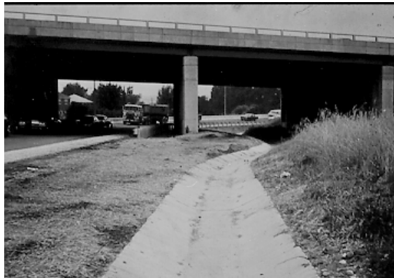
Figure 30. Rigid concrete channel lining.
